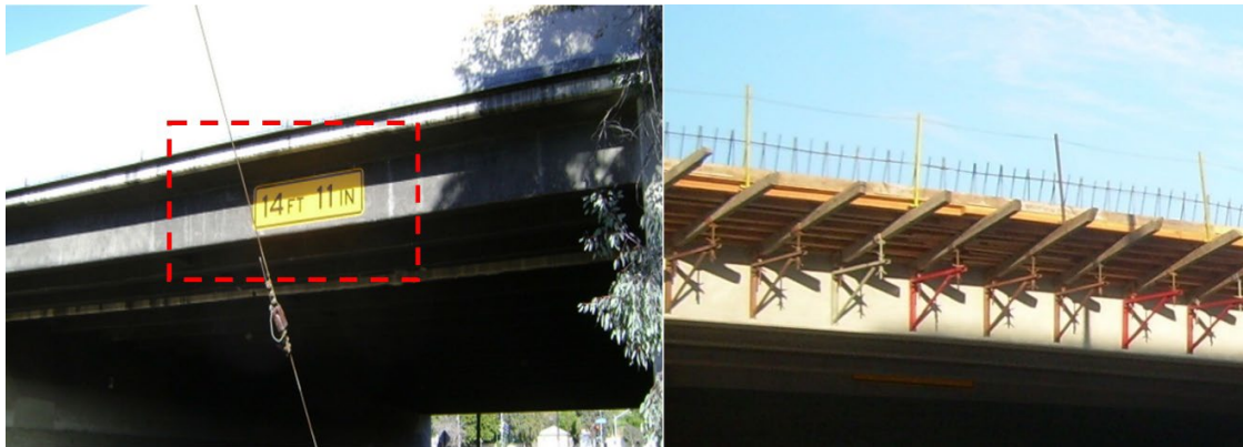
Figure 1-4. Example of a Field and Construction Conflict
