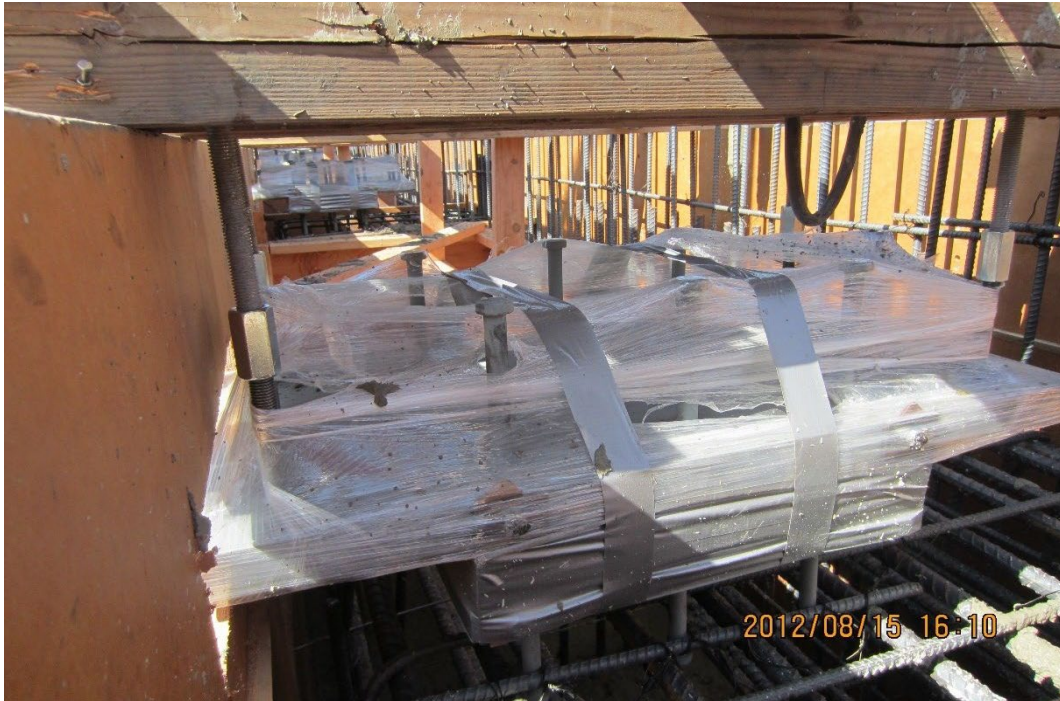
Figure C-1. Protective Measures Taken to Protect the PTFE from Concrete Intrusion During Concrete Placement (SFOBB Touchdown Project)
