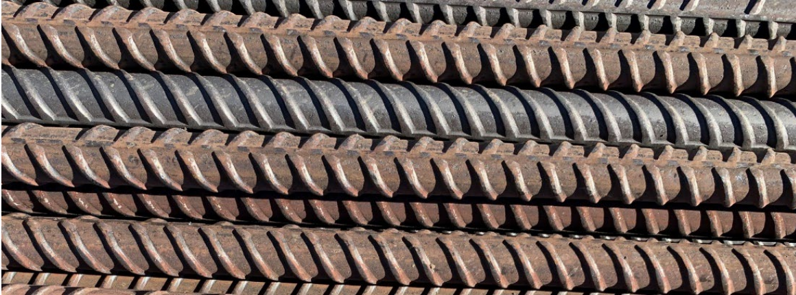
Figure 4-5. Light Rust on Bar Reinforcement
