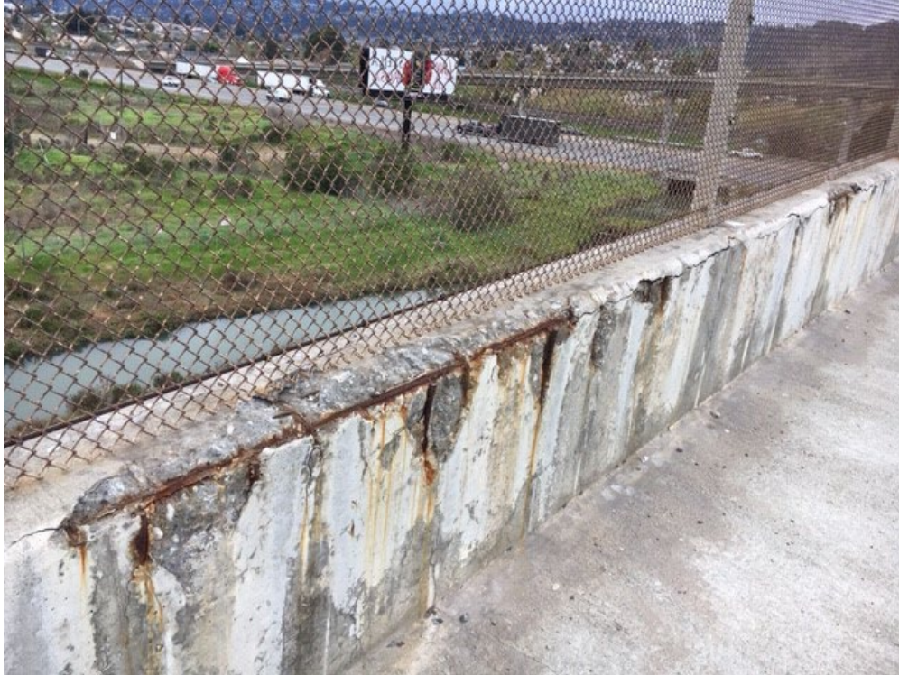
Figure 4-8. Bar Reinforcement Rusting and Concrete Spalling on Barrier
