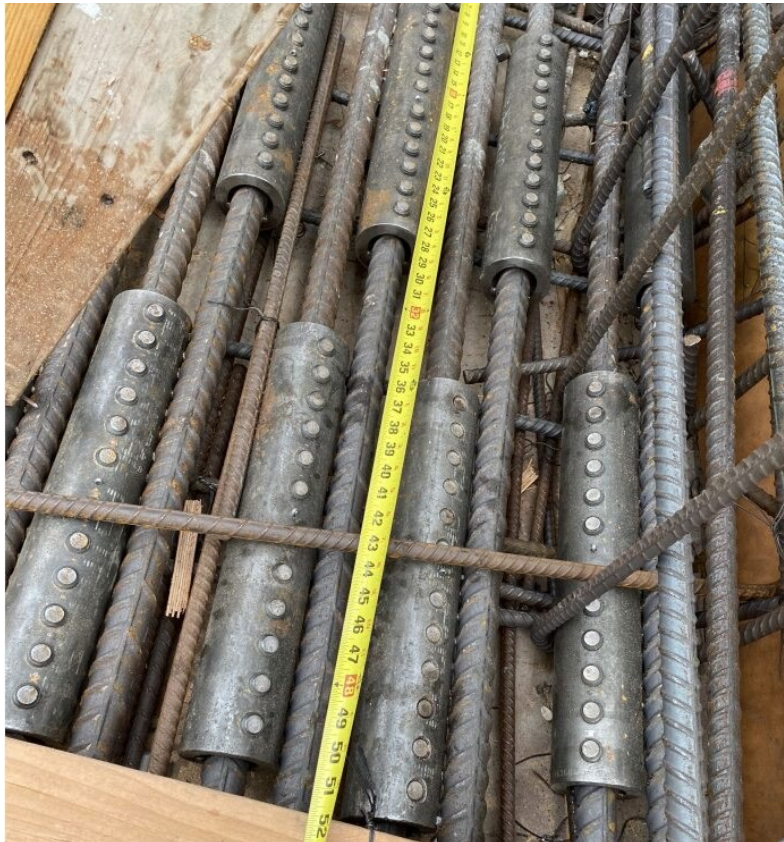
Figure 4-16. Congestion of Mechanical Couplers
