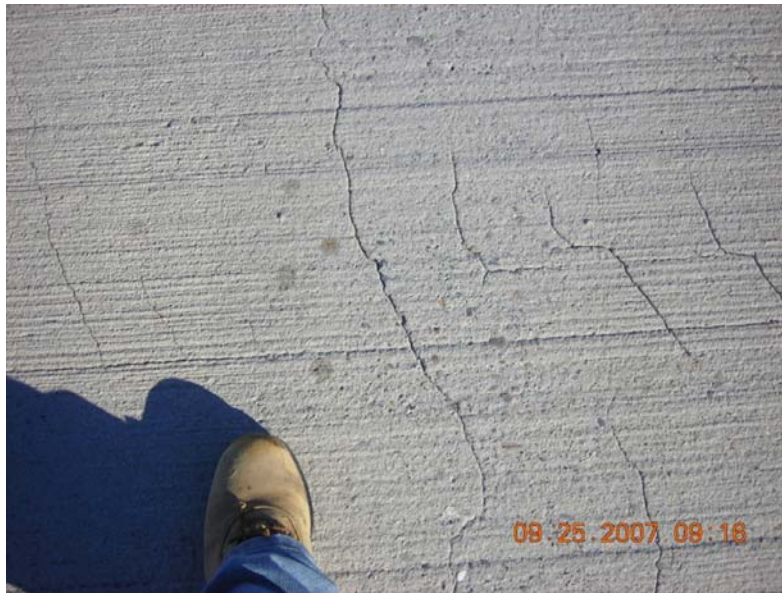
Figure No. 1: Example of Plastic Cracks on the Bridge Deck Surface
