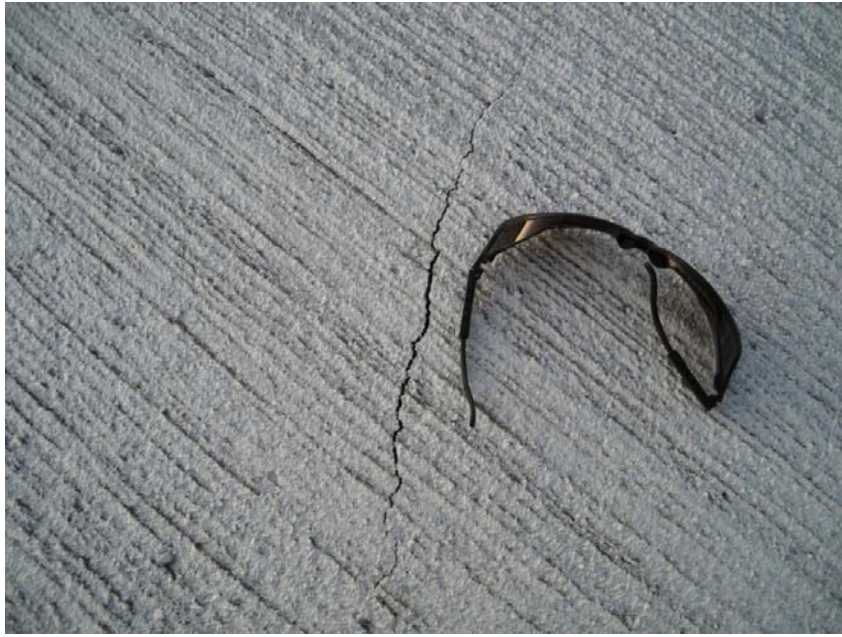
Figure No. 2: Example of Plastic Cracking Occurring After Curing Compound Application.
