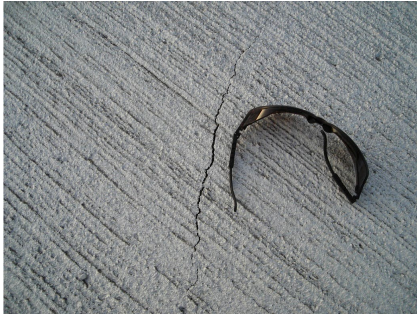
Figure 2. Example of Plastic Cracking Occurring After Curing Compound Application
