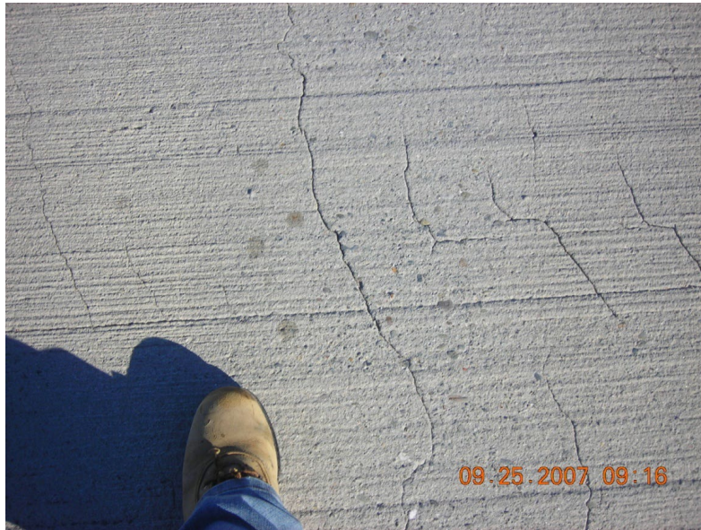
Figure 1. Example of Plastic Cracks on the Bridge Deck Surface
