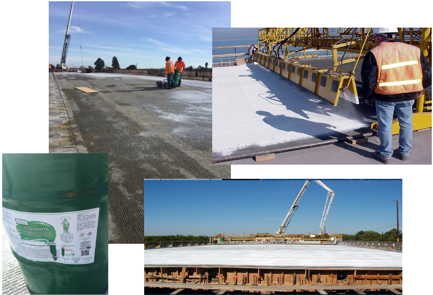
Figure 9. Remove curing medium and apply curing compound during the same work shift
