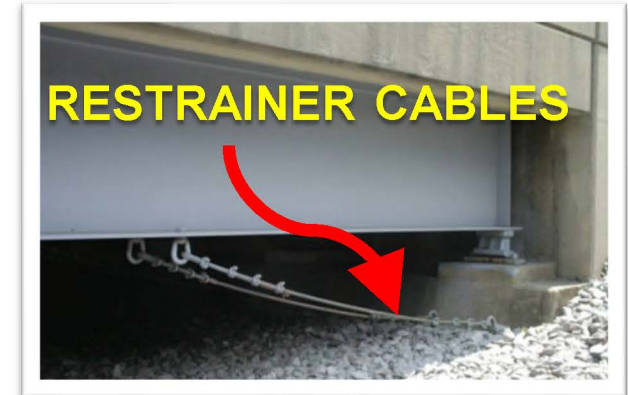
HWY BRIDGES: Restrainer to protect the bridge
