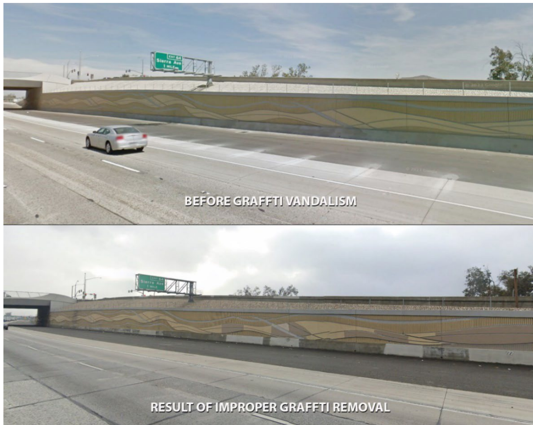
Figure 2.8.11-1 Undesired Result from Painting Over Graffiti
