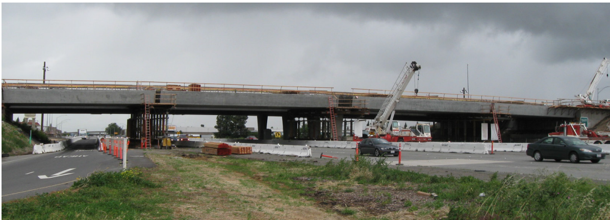
Figure 5.3.3-8 Precast Bath-tub Girder Segments Spliced Near Midspan Using Temporary Supports at Harbor Blvd. Overcrossing (Bridge No. 22-0108, Caltrans)
