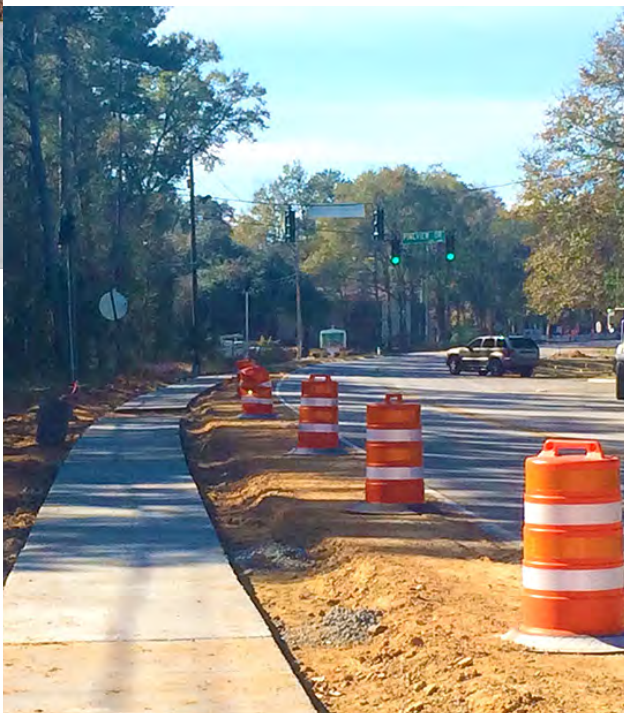
A sidewalk installation on a rural route as part of a "Safe Route to School" initiative. Photo credit: Valdosta-Lowndes MPO, Flickr CCL.
