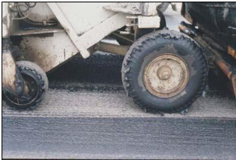
Figure 8-10. Tack coat tracking resulting in no tack coat in the wheel path.
