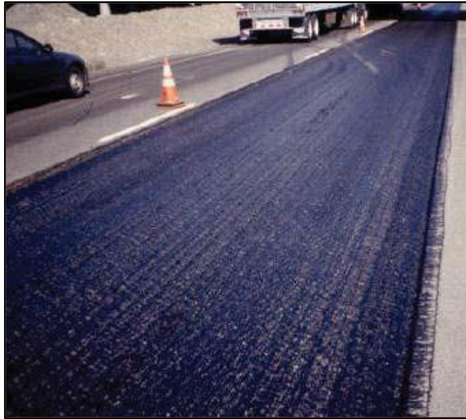
Figure 8-9. Tack coat using an asphalt emulsion. The black color indicates it has broken.
