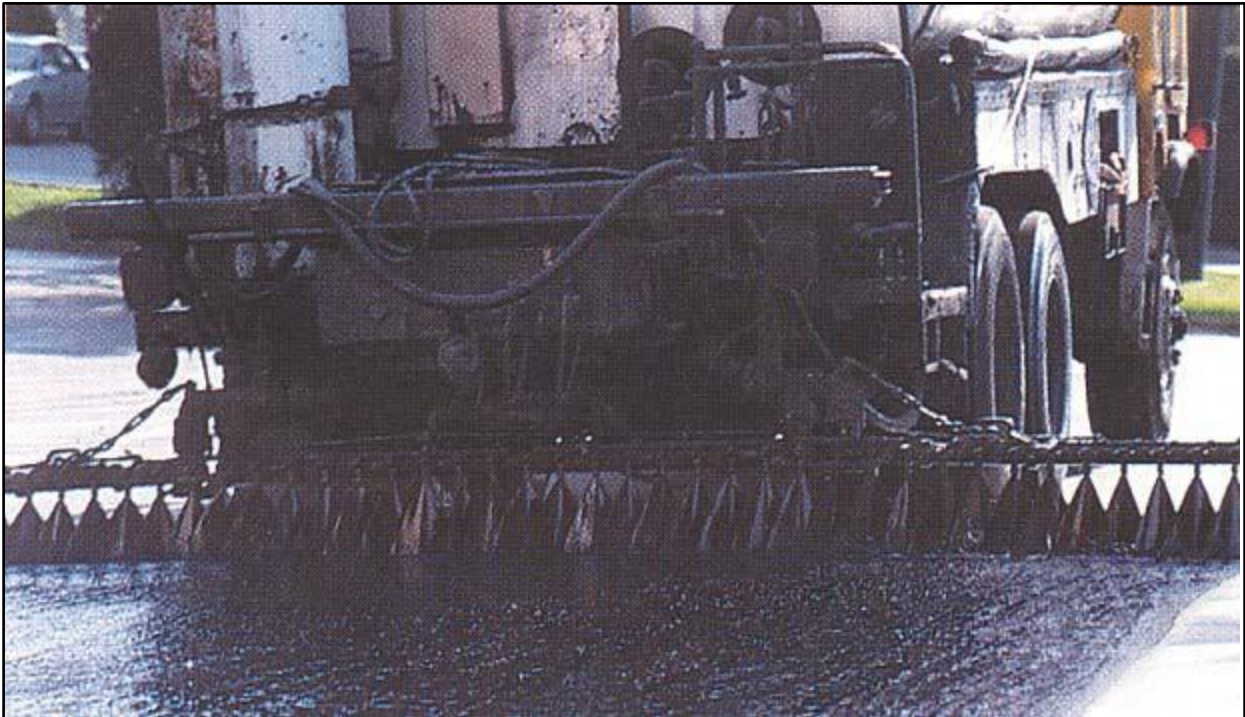
Figure 8-2. Set the height of the spray bar high enough above the roadway for the surface to receive double or triple coverage.
