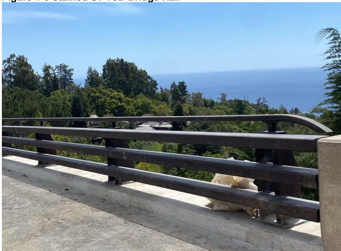
Figure 1-3 Stained ST-75B Bridge Rail
