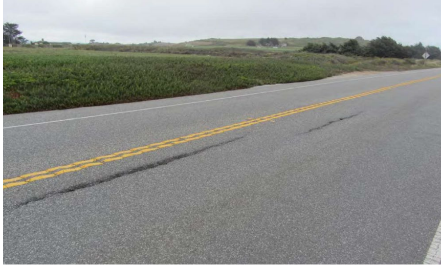
Figure 1-4. Cracks Running Longitudinally to the Roadway Surface. These areas are also indicators of subsurface failure of the support of the roadway surface due to erosion occurring at the bluffs and under the roadway embankment.
