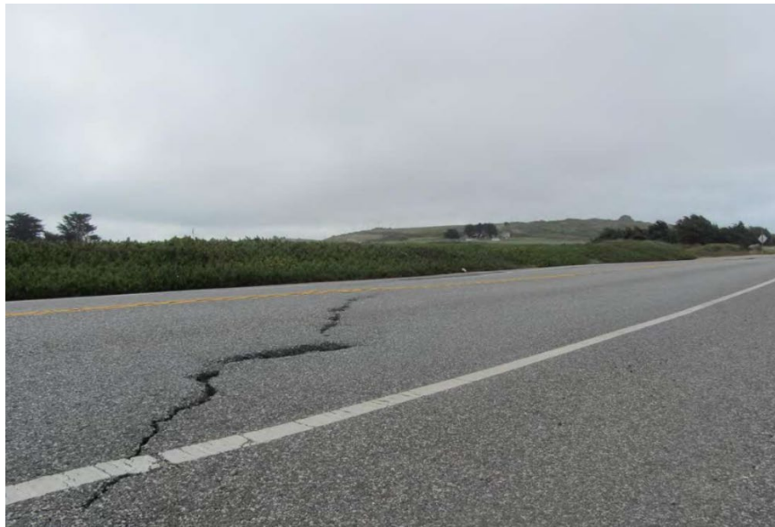
Figure 1-3. Roadway Cracking. This figure shows cracks running along the roadway surface, a symptom of underlying erosion occurring below the surface of the roadway.
