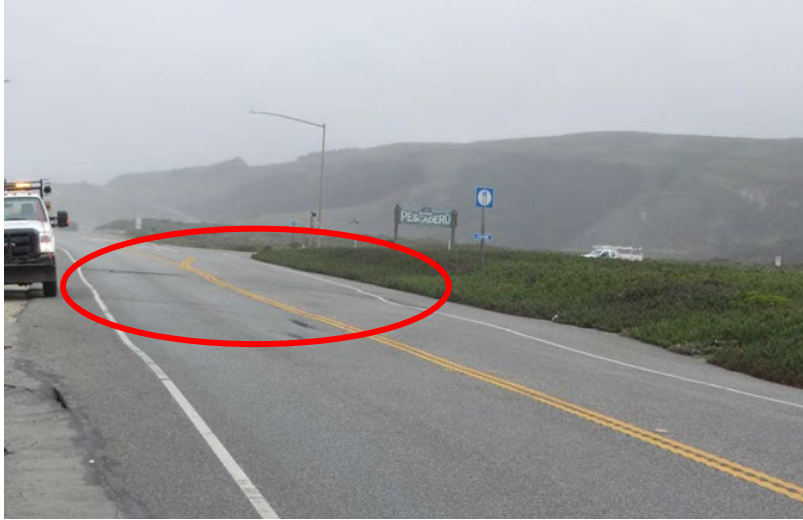
Figure 1-2. Roadway Depression. This figure shows a roadway depression where the road surface and underlying support is sinking due to erosion occurring below the roadway surface.
