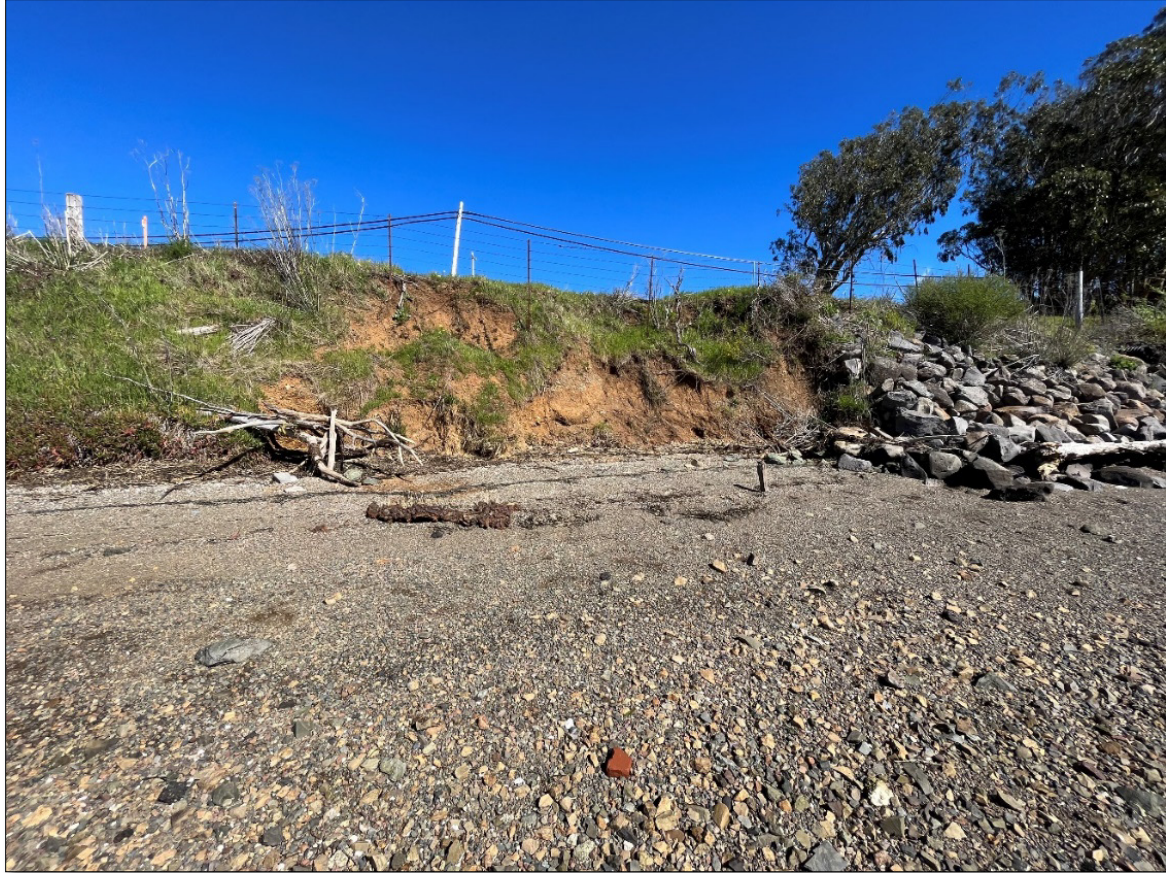
Figure 3. Eroded slope on southbound side of SR 1.
