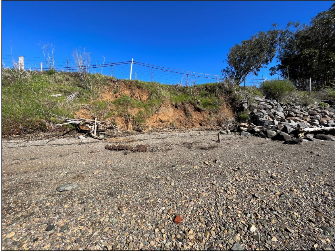
Figure 3. Eroded slope on southbound side of SR 1.
