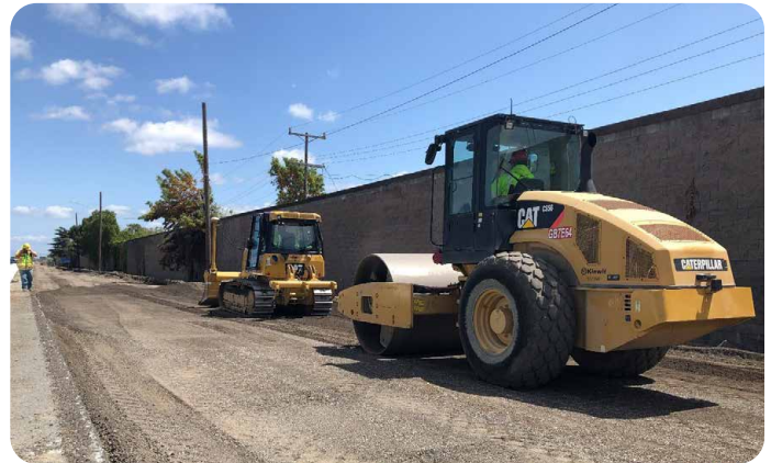
Construction crews leveling a new section of freeway shoulder in Phase Two.
