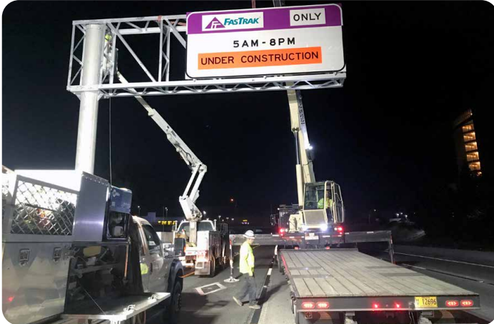
Construction crews installing a new overhead sign in the median in Phase One.
