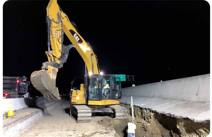
Construction crews excavating on a section of freeway shoulder. Crews are excavating, grading, and paving to create a new lane on each side of the freeway from Whipple Avenue to I-380 in Phase Two.
