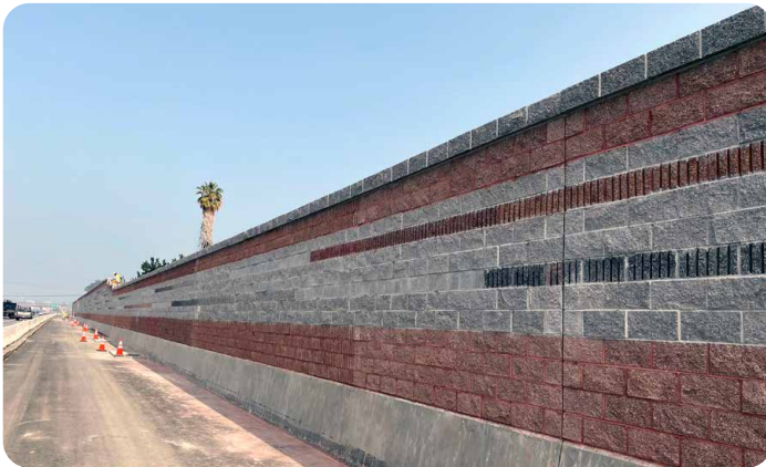
Completed section of sound wall on Bayshore Boulevard from Dore Avenue to East Poplar Avenue in the City of San Mateo.
