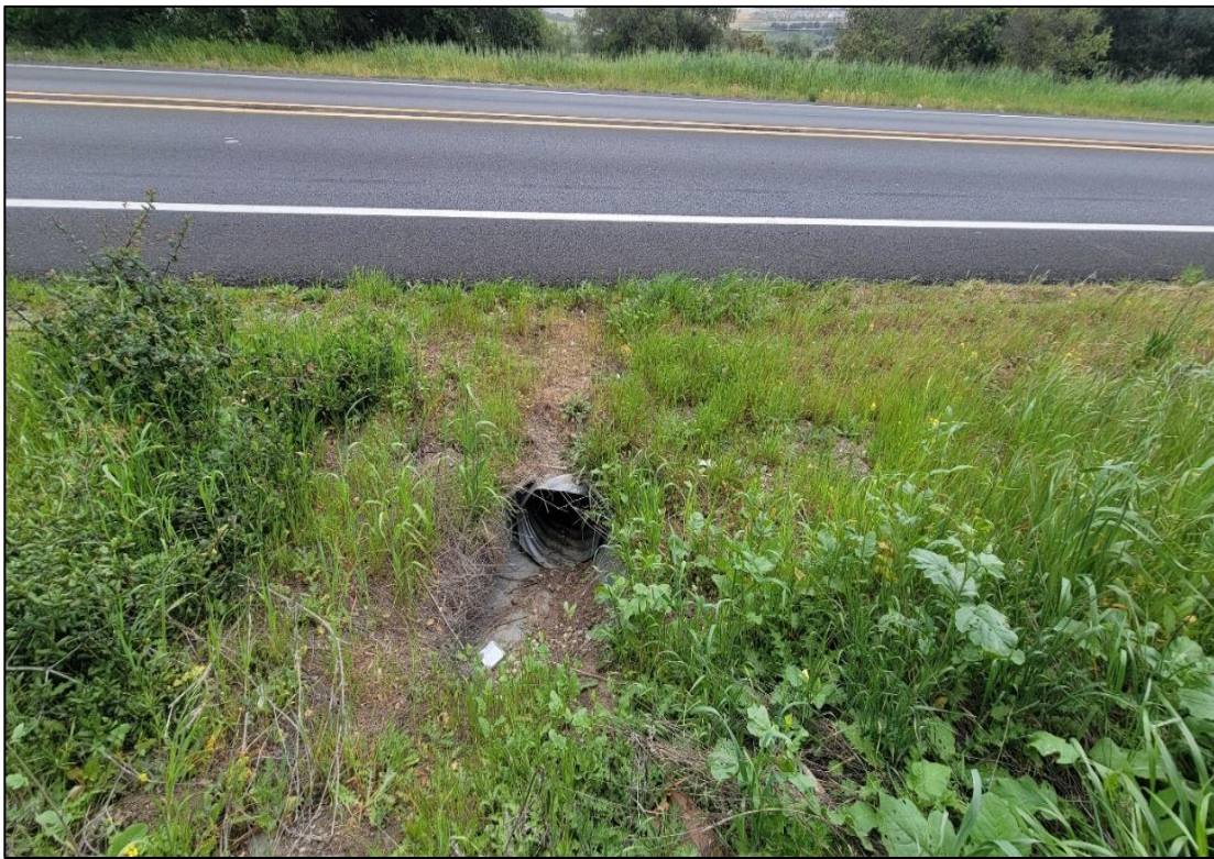
Figure 4. Proposed drainage location #1 along WB SR 74, PM 3.6 (Qya deposits), view south.
