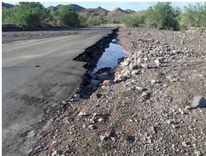
EROSION ON HIGHWAY 78
