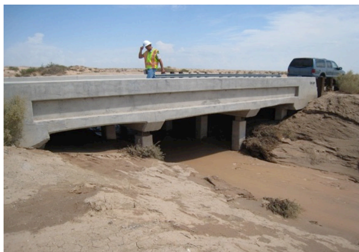
HIGH FLOWS UNDER BRIDGE ON SR-78
