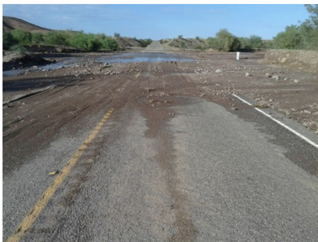
FLOODING ON HIGHWAY 78
