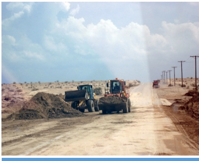
REPAIRS TO SR-78 ROADWAY AFTER STORM DAMAGE
