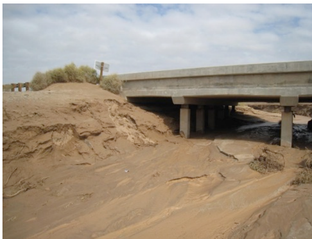
SR-78 STORM DAMAGE
