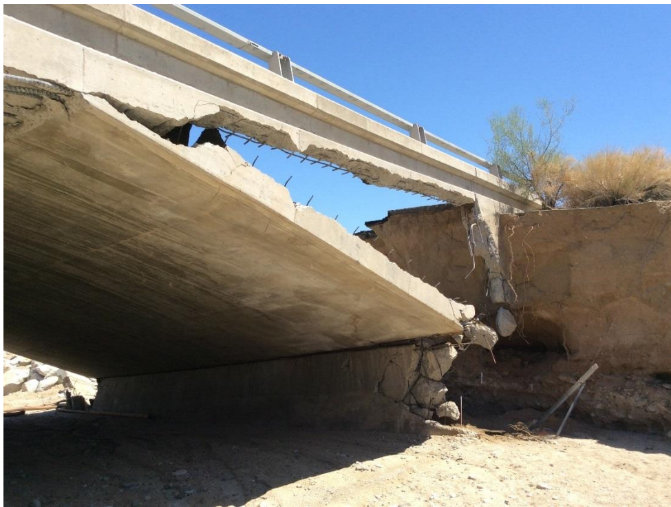
FIGURE 20: TEX WASH BRIDGE ABUTMENT AND DECK COLLAPSE
