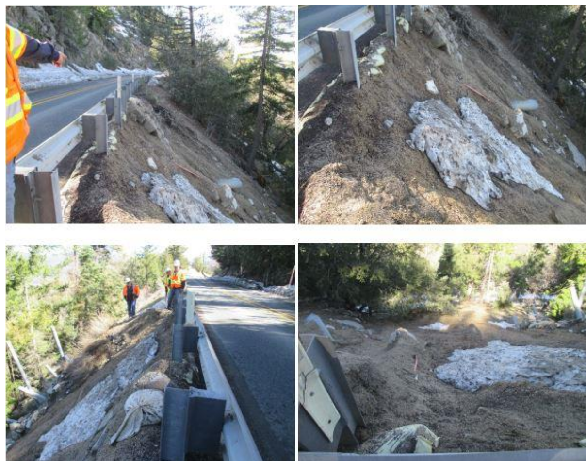
FIGURE 6: SLOPE DEGRADATION ON SR-38
