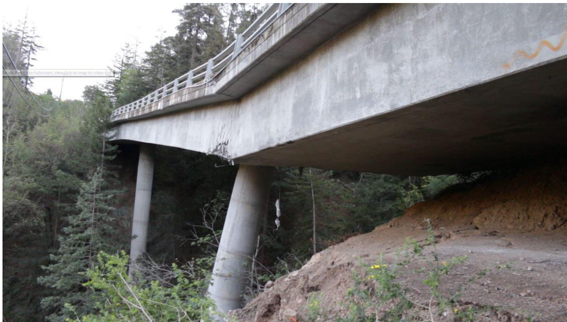
FIGURE 2: US 1 PFEIFFER CANYON DAMAGED BRIDGE, 2017
