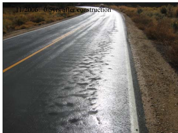
Figure 4.60: Roughness in asphalt concrete on 07-VEN-33.
