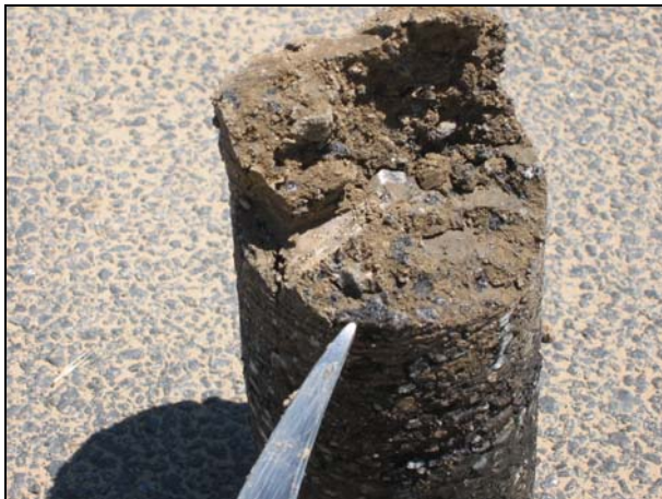
Figure 4.32: Core showing fines contamination. (2)
