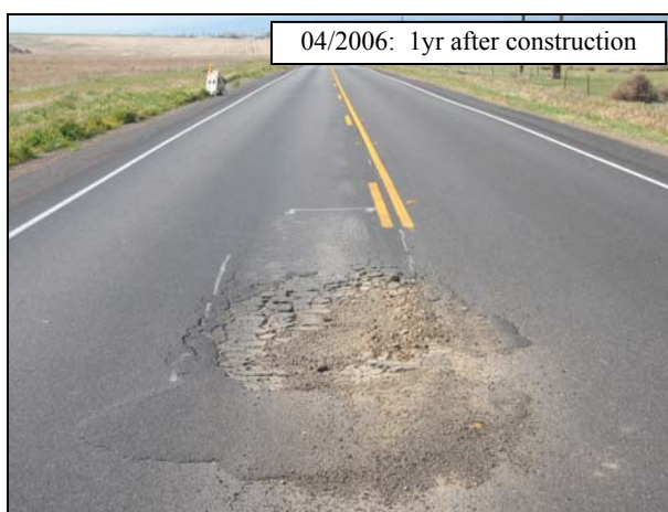
Figure 4.13: Severe distress (1) on 05-SB,SLO-33 (April 2006).
