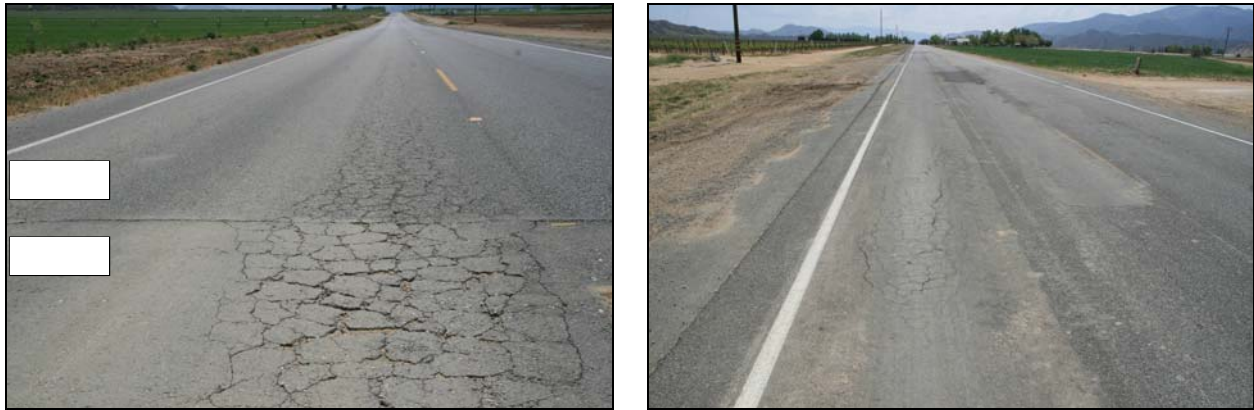
Figure 4.27: New distress on previous digout on 05-SB,SLO-33 (May 2008).
