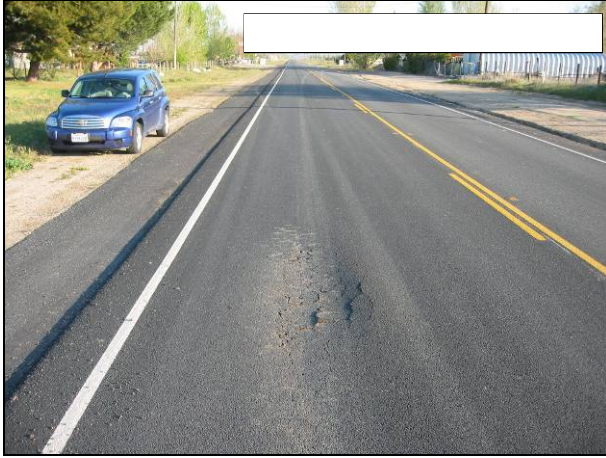
Figure 4.14: Severe distress (2) on 05-SB,SLO-33 (April 2006).
