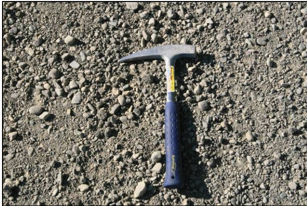
Figure 7.34: Poor surface compaction in areas of recycling in cold temperatures.
