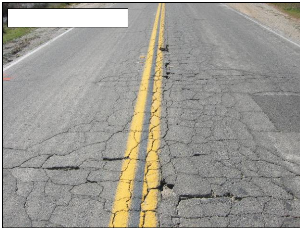
Figure 4.34: Preconstruction fatigue (alligator) cracking on 07-VEN-33.
