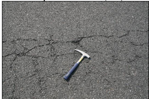
Figure 4.5: Spalled cracks through open-graded friction course on 03-COL-20 (2008).
