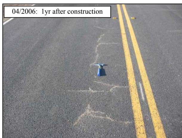
Figure 4.12: Early cracking with pumping on 05-SB,SLO-33 (April 2006).
