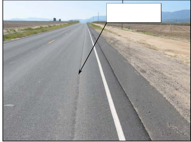
Figure 4.23: Construction defect on 05-SB,SLO-33.
