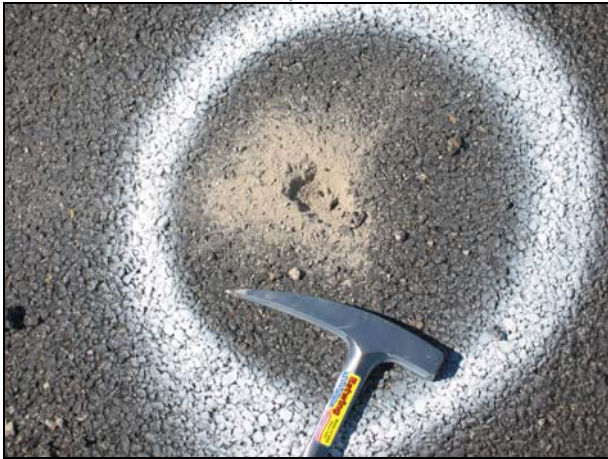
Figure 4.24: Area of thin asphalt concrete on 05-SB,SLO-33.
