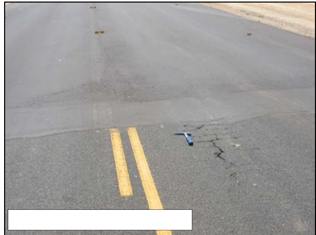
Figure 4.17: New distress next to digout on 05-SB,SLO-33 (July 2006).
