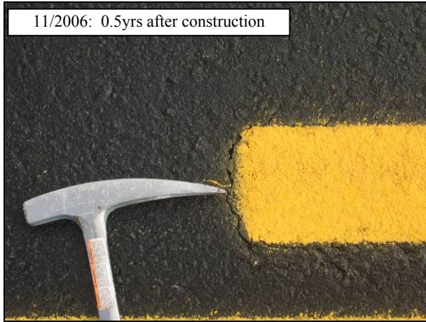
Figure 4.61: Cracking around centerline striping on 07-VEN-33.
