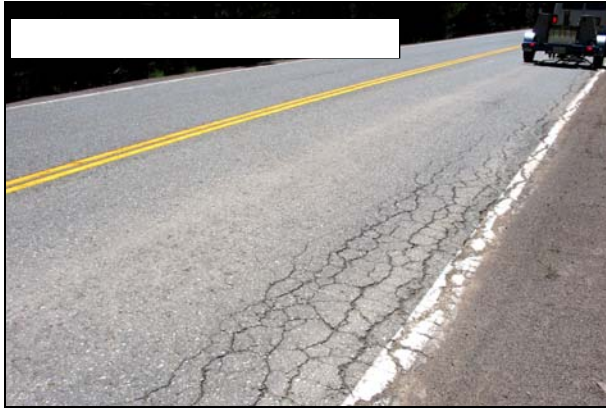
Figure 4.7: Outer wheelpath cracking on 03-SIE-89.
