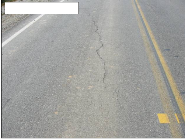
Figure 4.36: Preconstruction longitudinal cracking on 07-VEN-33.
