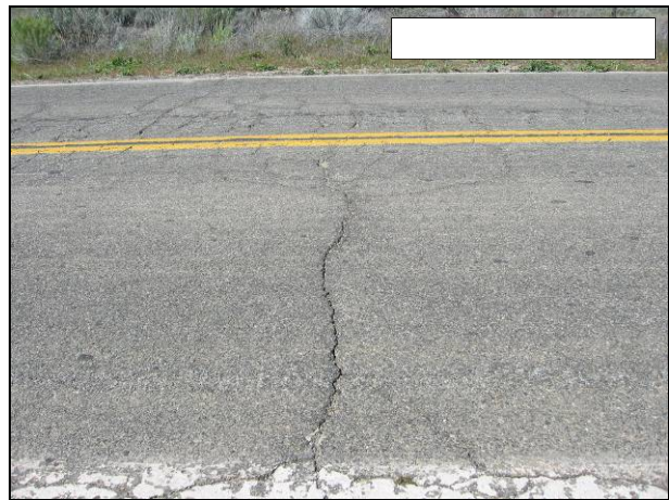
Figure 4.35: Preconstruction transverse cracking on 07-VEN-33.
