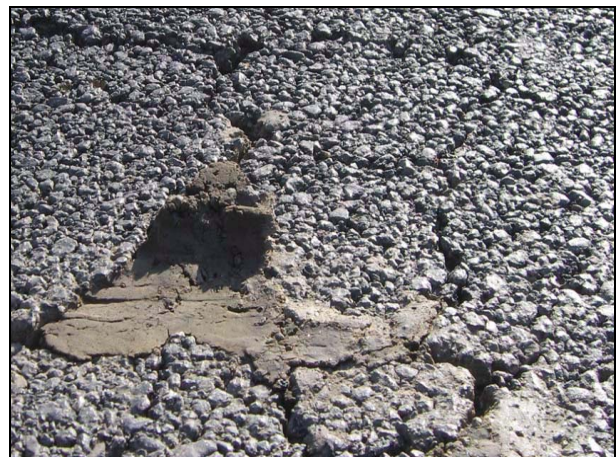
Figure 4.33: Fines pumped through base and asphalt concrete.
