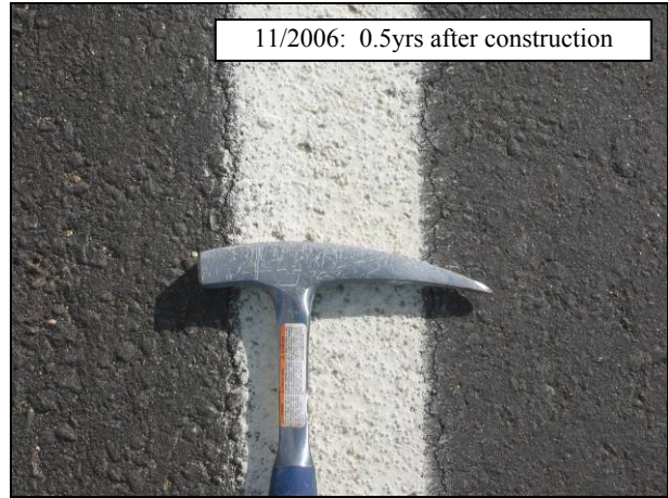
Figure 4.62: Cracking around edge striping on 07-VEN-33.
