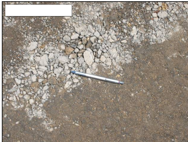
Figure 4.54: Area of segregated aggregate on 07-VEN-33.
