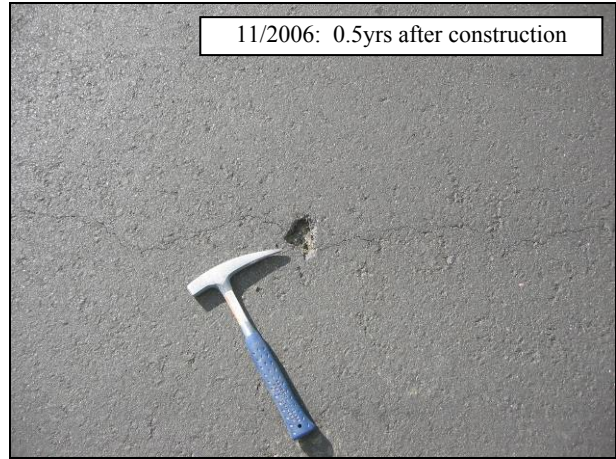
Figure 4.57: Longitudinal crack and loss of oversize stone on 07-VEN-33.
