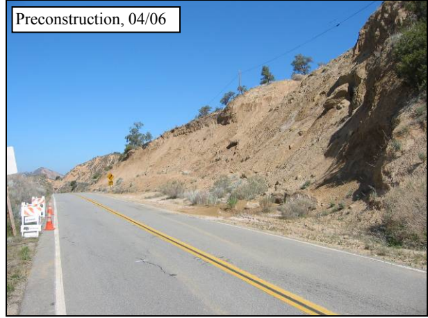
Figure 4.37: Preconstruction cracking associated with slope instability on 07-VEN-33.
