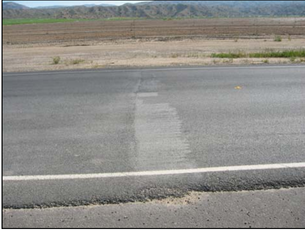
Figure 4.22: Poor construction joint on 05-SB,SLO-33.
