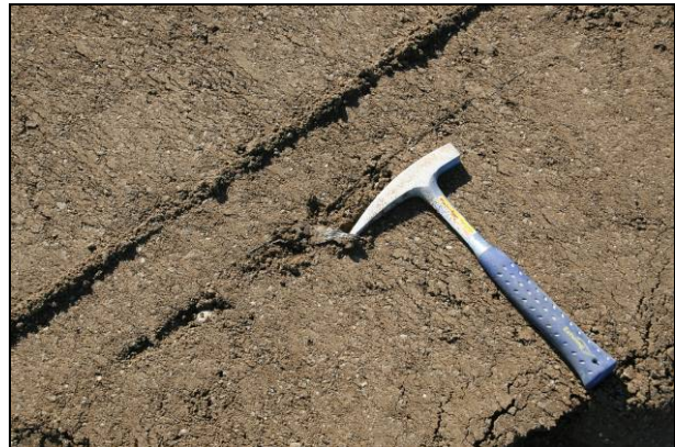
Figure 7.31: Asphalt strings in recycled material.
