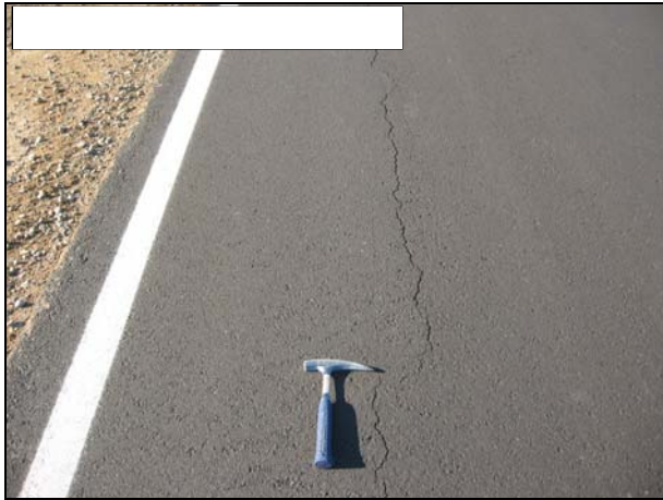
Figure 4.66: Longitudinal cracking on 07-VEN-33 (April 2007).
