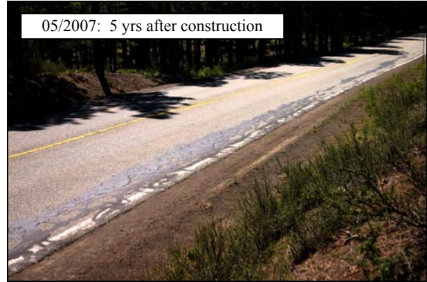
Figure 4.8: Sealed outer wheelpath cracks on 03-SIE-89.
