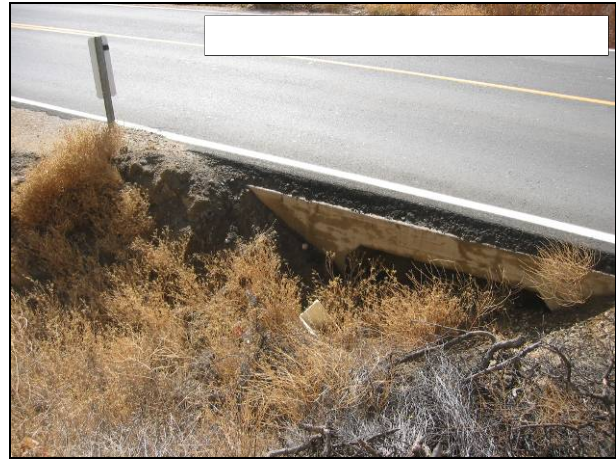
Figure 4.64: Blocked drain. (1) on 07-VEN-33.
