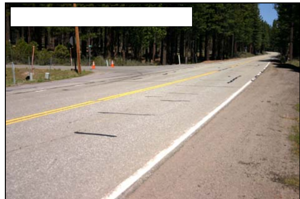
Figure 4.10: Sealed transverse cracks on 03-SIE-89.
