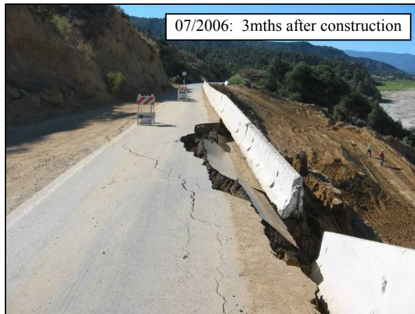
Figure 4.68: Damage associated with landslide (July 2006).
