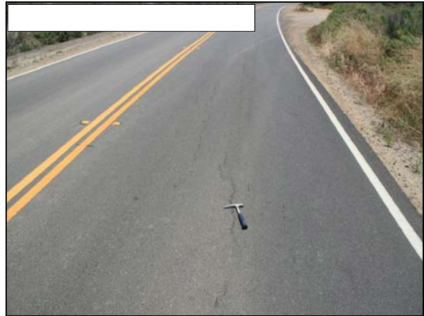
Figure 4.67: Longitudinal cracking on 07-VEN-33 (May 2008).
