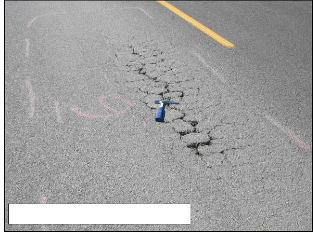
Figure 4.15: Severe distress (3) on 05-SB,SLO-33 (July 2006).
