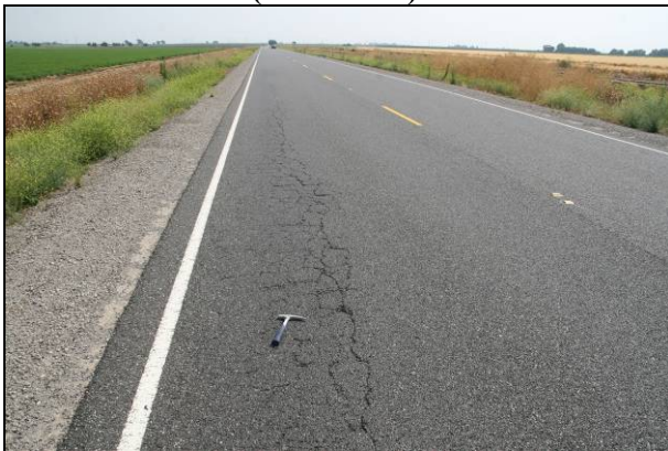
Figure 4.4: Fatigue cracking in outer wheelpath on 03-COL-20 (2008).
