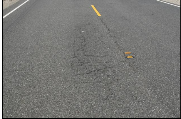
Figure 4.3: Fatigue Cracking in inner wheelpath on 03-COL-20 (2007).
