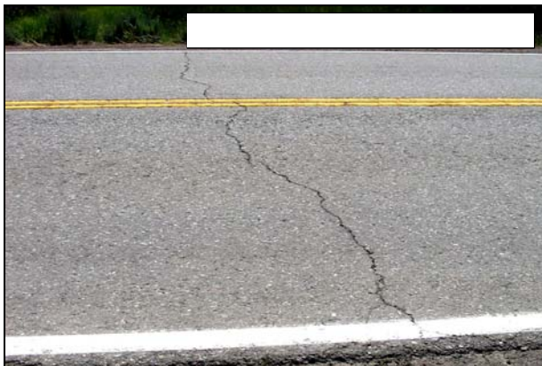
Figure 4.9: Thermal cracking on 03-SIE-89.
