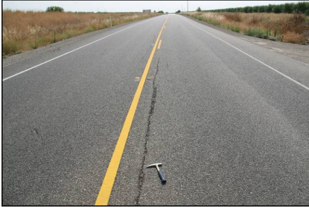
Figure 4.2: Centerline crack on 03-COL-20 (2006–2008).
