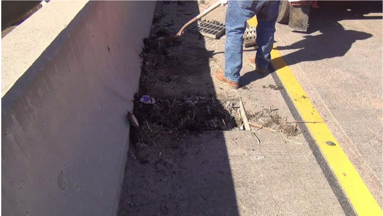
Figure 5.2: Shoveling debris downstream of the grate for the sweeper to pick up
