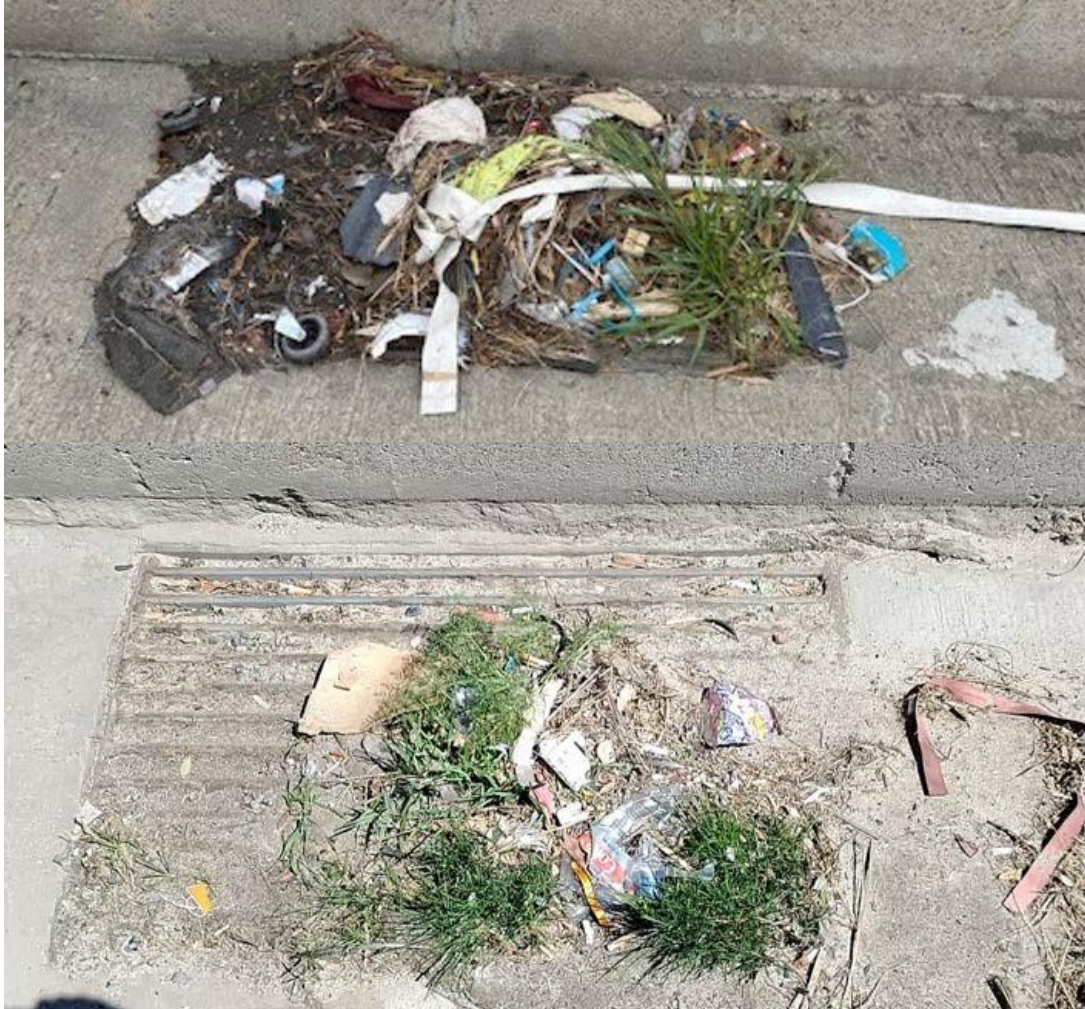
Figure 3.1: Two examples of debris-filled grates (Images from District 11)
