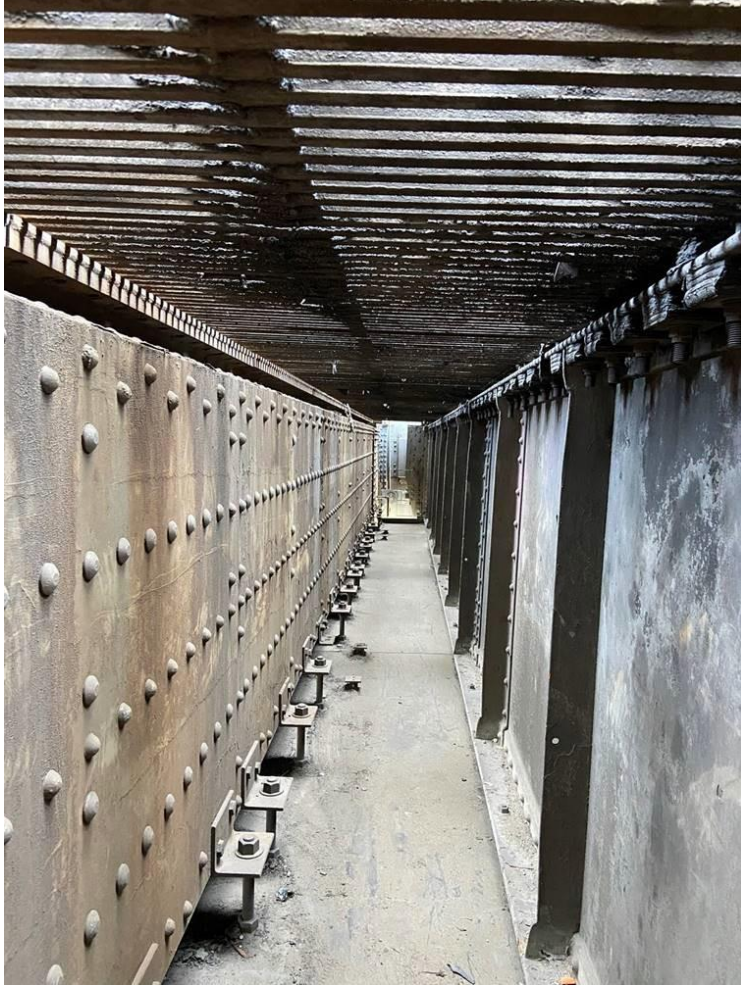
Figure 3.4: Bay Bridge pan that is cleaned by hand every six months (Image from Caltrans District 4)
