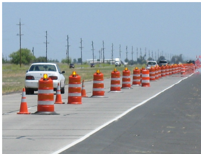
Image 3: Warning Lights on SR52 Los Banos, CA
