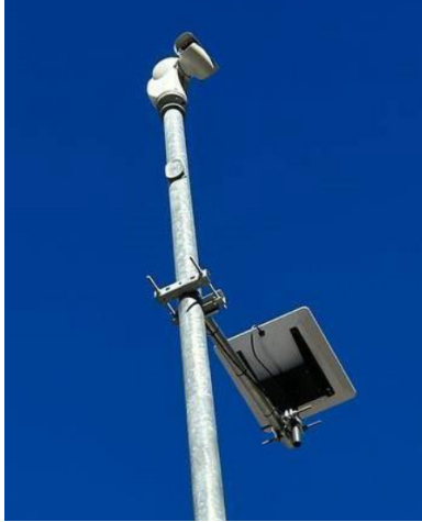
Image 3: Starlink high-performance flat antenna after installation – Image Source – AHMCT
