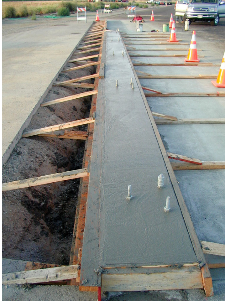
Figure 2-6 - Curb Concrete with Protruding Post Bolts
