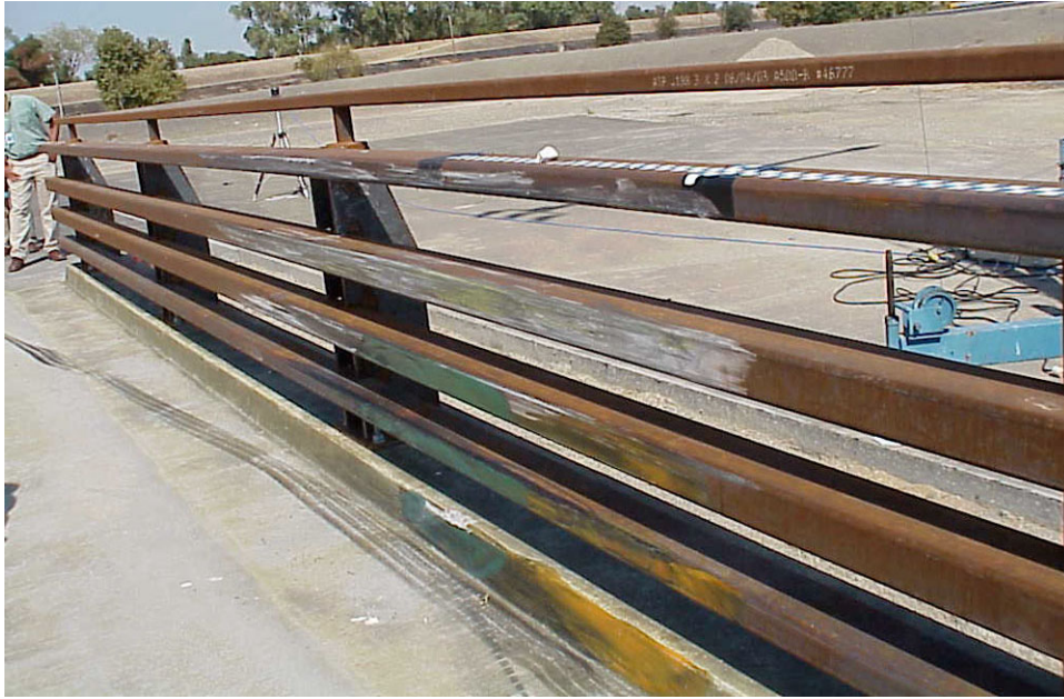
Figure 2-17 - Test 651 Rail Scuffing
