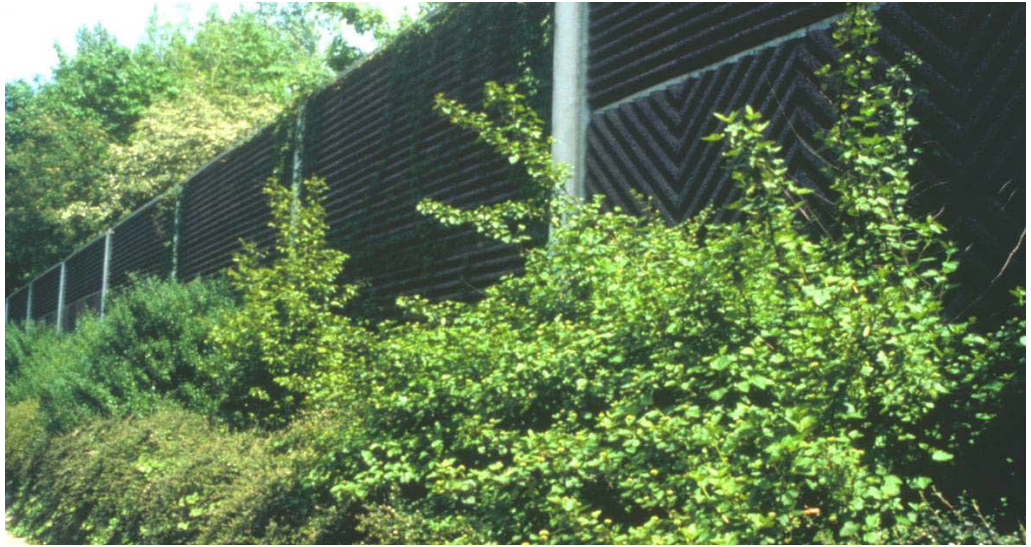
Figure 1.5. 4 m high profile brown concrete noise barriers with 1 m high plant box for vegetation along Highway A4 southeast of Cologne, Germany [3].
