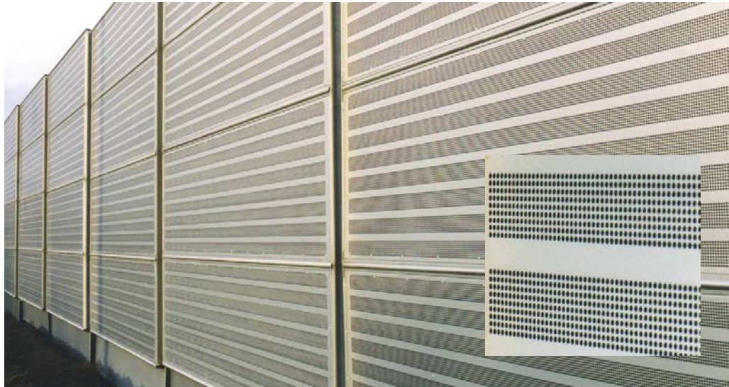
Figure 2.14. Noise absorbing steel barrier with perforated surface and absorbing material at a highway in Denmark (close up to the right) [2].
