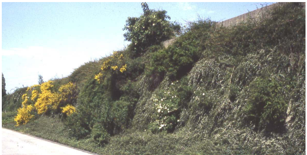
Figure 3.23. 7 m (23 ft.) high supported earth embankment with vegetation along Highway A3 near Cologne, Germany [3].
