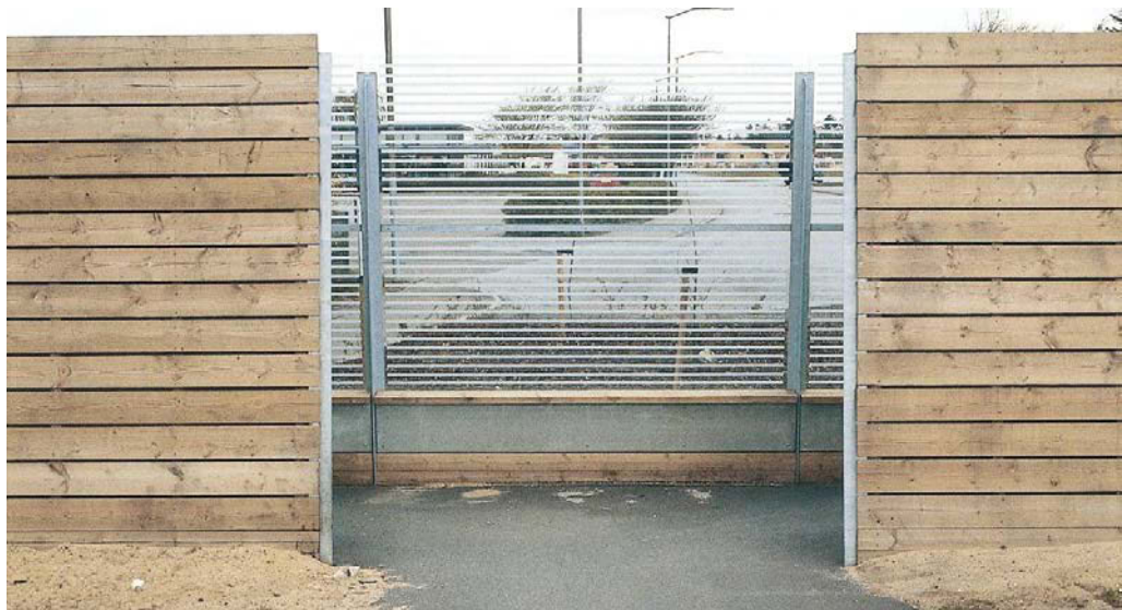
Figure 2.7. 2.5 m high wooden noise barrier in Denmark with passage for pedestrians and bikes at National Road 411 in Skive. A transparent barrier is used behind the wooden barrier to create a noise sluice [1].
