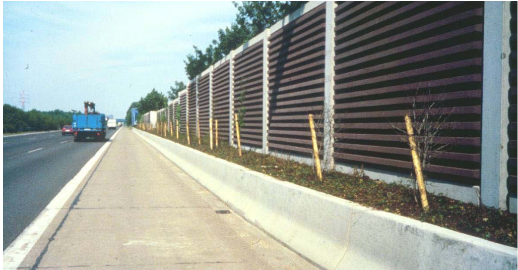
Figure 3.19. 4 m (13 ft) high brown profiled concrete noise barrier with 1 m high plant box with new vegetation in the front at Highway A4 in Germany [3].
