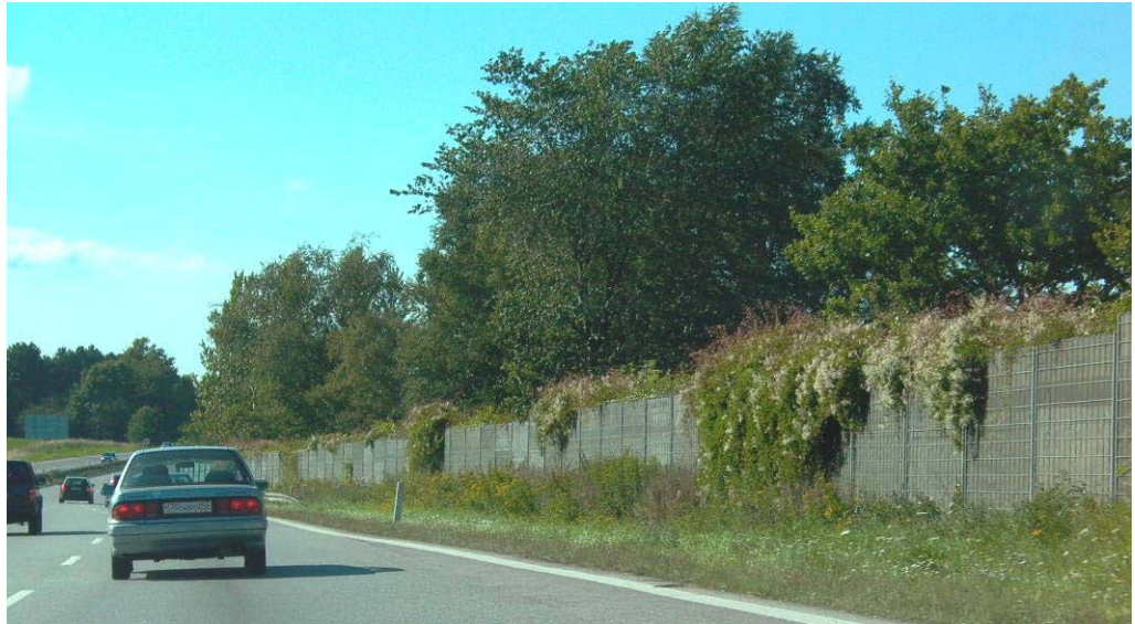
Figure 2.13. Absorbing noise barrier with vegetation at Highway M14 north of Copenhagen, Denmark.
