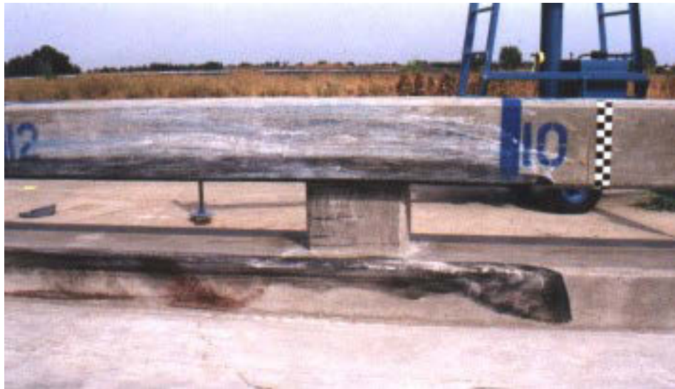
Figure 2-20 Post Impact Bridge Rail Scuff Marks Test 544
