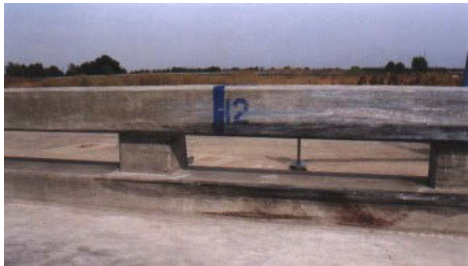
Figure 2-21 Post Impact Bridge Rail Scuff Marks Test 544
