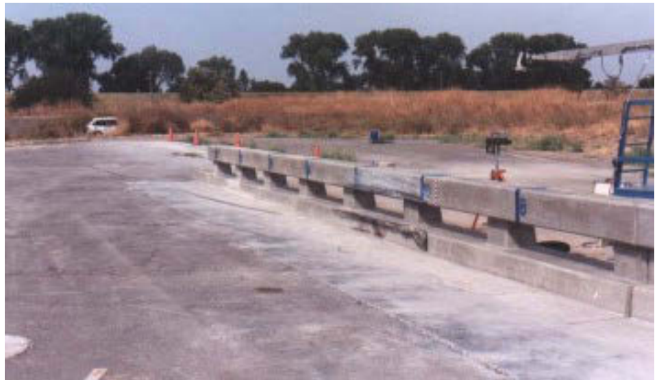
Figure 2-19 Post Impact View of Barrier and Vehicle 544
