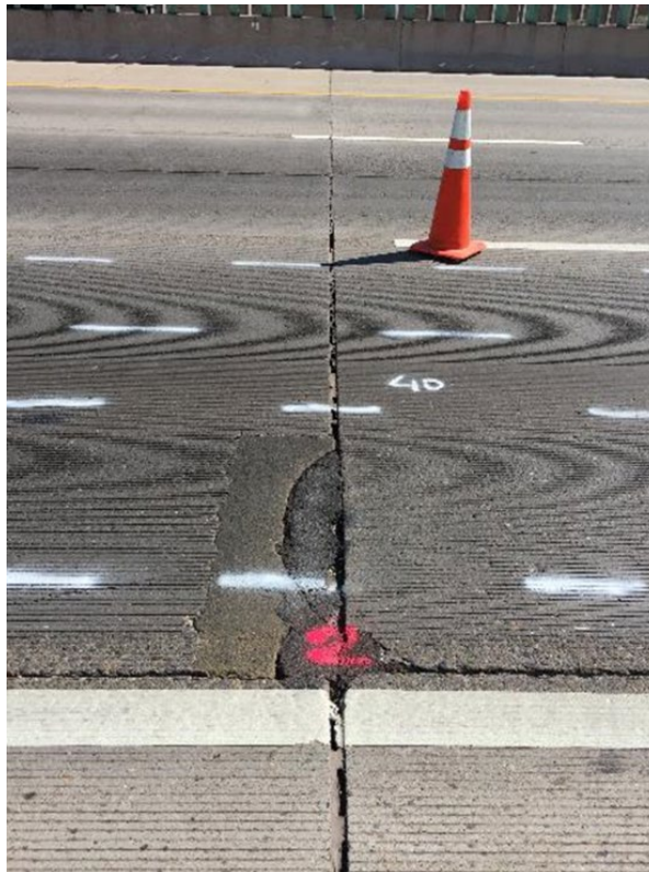
Figure 15. Example marking of joints (red #2) and intermediate points (40 ft. station mark) on jointed concrete pavement.
