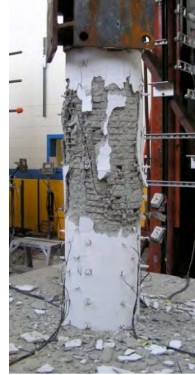
(b) Axial failure of the column
