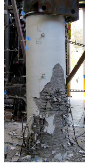
(b) Axial failure of the column
