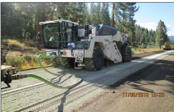
Figure 3.18: PLU147: Water pipe dragging on cement.
