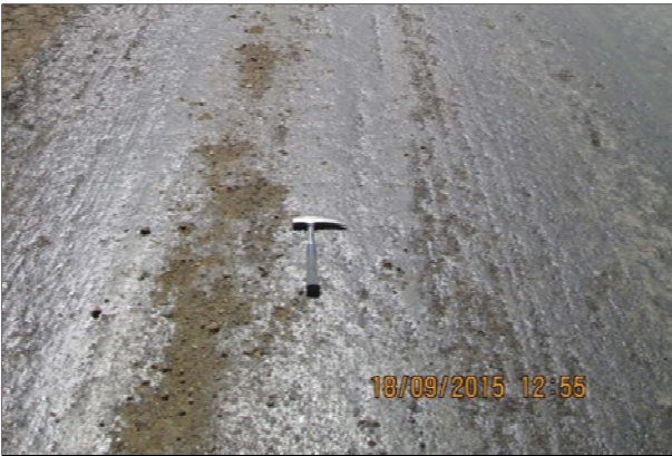
Figure 3.16: PLU147: Prime coat stripped from FDR-PC layer after traffic.
