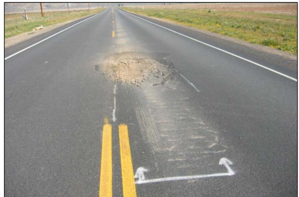
Figure 2.6: Pumping through fatigue cracking.
