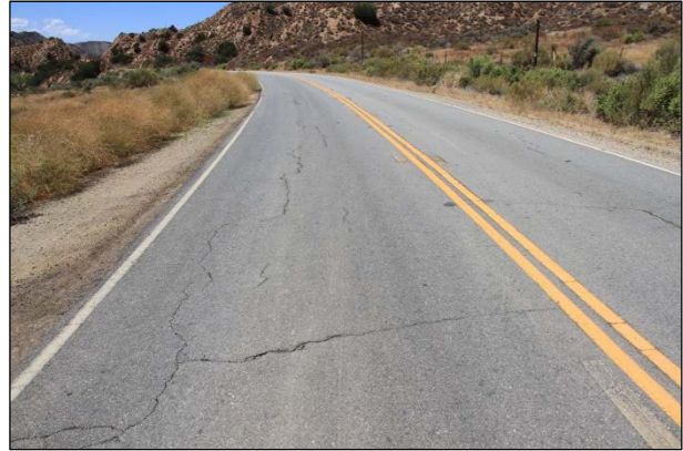
Figure 2.4: Block crack progression.
