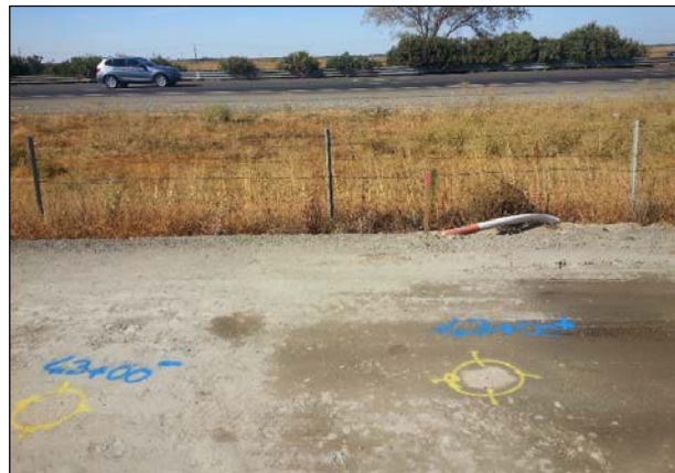
Figure 3.7: CR32B: Wet and adjacent dry locations tested with SSG.
