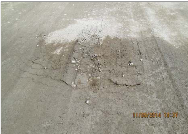
Figure 3.6: CR32B: Wet, soft location after final compaction.
