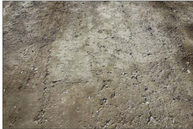
Figure 3.3: CR32B: Block cracking on FDR-PC prior to surfacing.
