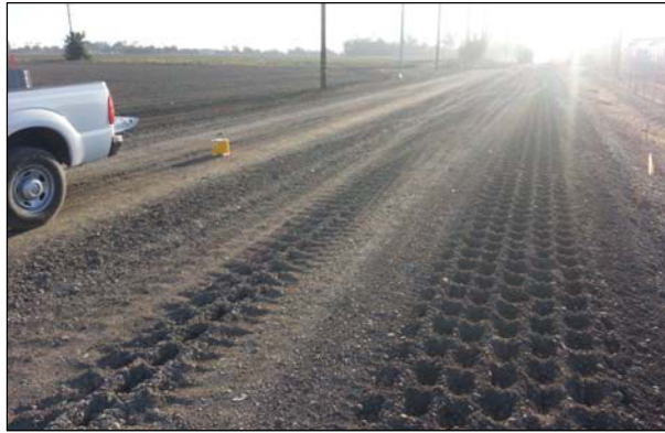
Figure 3.9: CR27: Incomplete compaction prior to start of next day construction.
