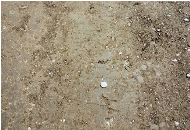
Figure 3.2: CR32B: Transverse cracking after microcracking.
