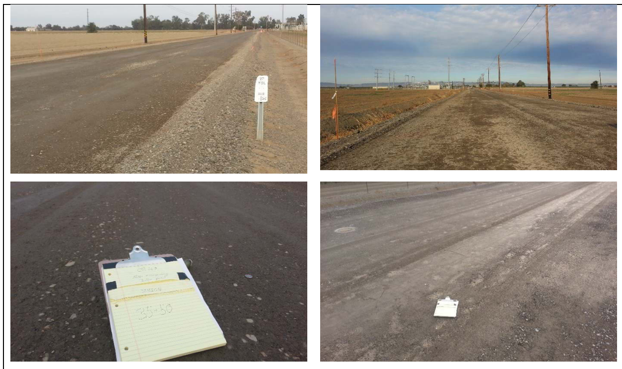
Figure 3.32: CR27: Photographs showing wet surface.
