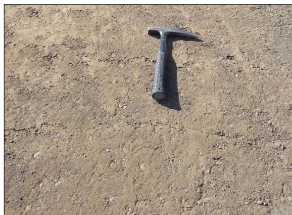
Figure 3.15: CR99: Block cracking after microcracking.
