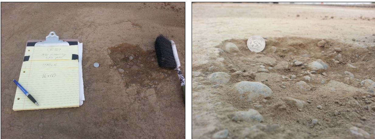
Figure 3.12: CR27: Distressed surface of FDR-PC layer after microcracking near start of project.
