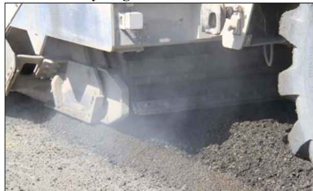
Figure 3.7: FDR-NS: Smoke during pulverization.
