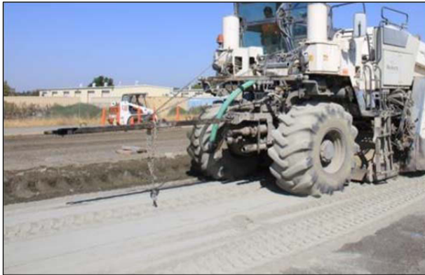
Figure 3.27: FDR-PC: Excess cement on Cell #7.
