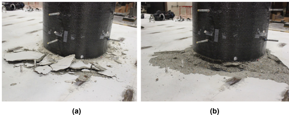
Figure 3.7 Damaged state of Specimen No. 2 (a) after all HS tests and (b) final view of this damage state after all loose concrete were removed.
