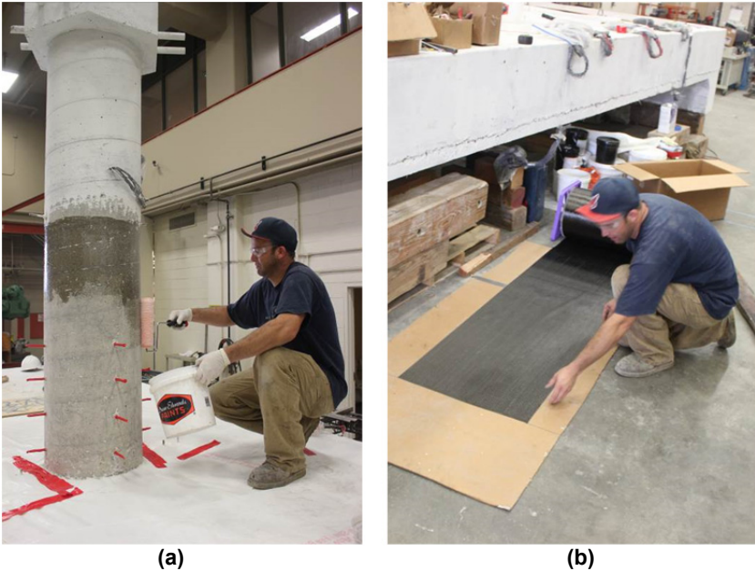
Figure 3.2 (a) Applying a primer epoxy coat to the column surface before applying the CFRP layers; and (b) preparing a single layer of a carbon fibers sheet and cutting the sheet to the desired length.
