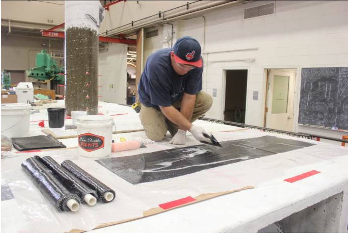
Figure 3.3 Coating the carbon sheets with epoxy resin and rolling the wet sheets in preparation for wrapping.
