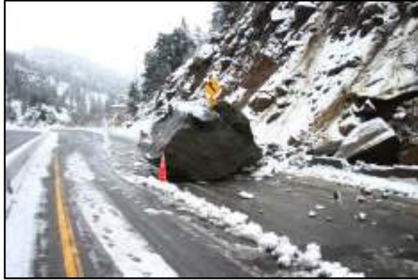
Figure 26. Large rockfall along U.S. 285 in Colorado that occurred in April 2007 (Photo courtesy of CDOT).
