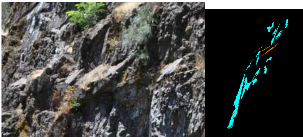
Figure 22. Left is an image of possible planar failure surfaces of approximately 50-degree dipping Joint Set 2 (light orange) with respect to the general rock face, while right shows a side view of Split-FX image of Joint Set 2 (orange) as compared to the main slope surface (teal).
