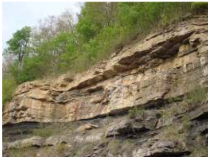
Figure 59. Photo of overhangs present on I-24 slope.
