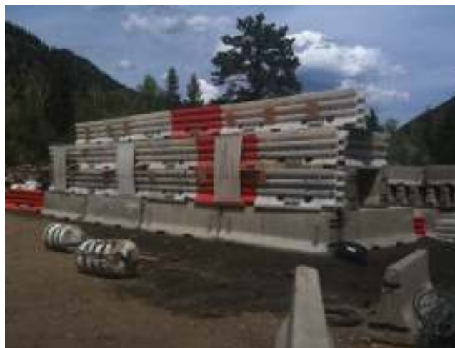
Figure 27a. At Site 2 in Colorado, an image of the jersey and plastic barriers.
