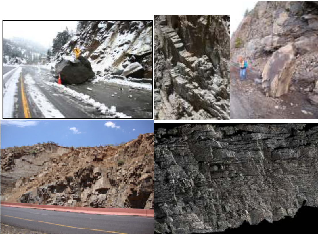
Figure 6. Images showing geotechnical issues associated with some of the pooled fund sites: top row, left to right, rockfall at one Colorado site, toppling at the California site, and rockfall at the Arizona site. Bottom left shows wedge failure at the Texas site, and bottom right shows overhangs at the New York site (Photos courtesy of CDOT).
