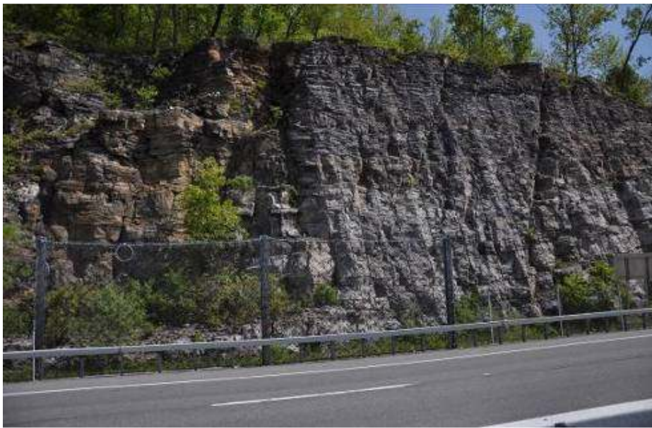
Figure 39. Southern section of rock slope at New York site showing the difference between pre-split (right) and conventional blasting (left).
