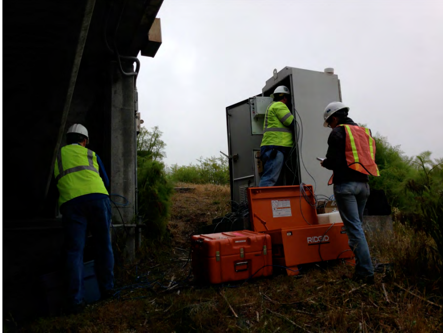
Figure 3-2: UCLA crew (R. Nigbor, S. Poulos) and the CGS technician (T. Shipman) are pictured while installing the Kinometrics Granite DAQ systems (photo by E. Taciroglu).
