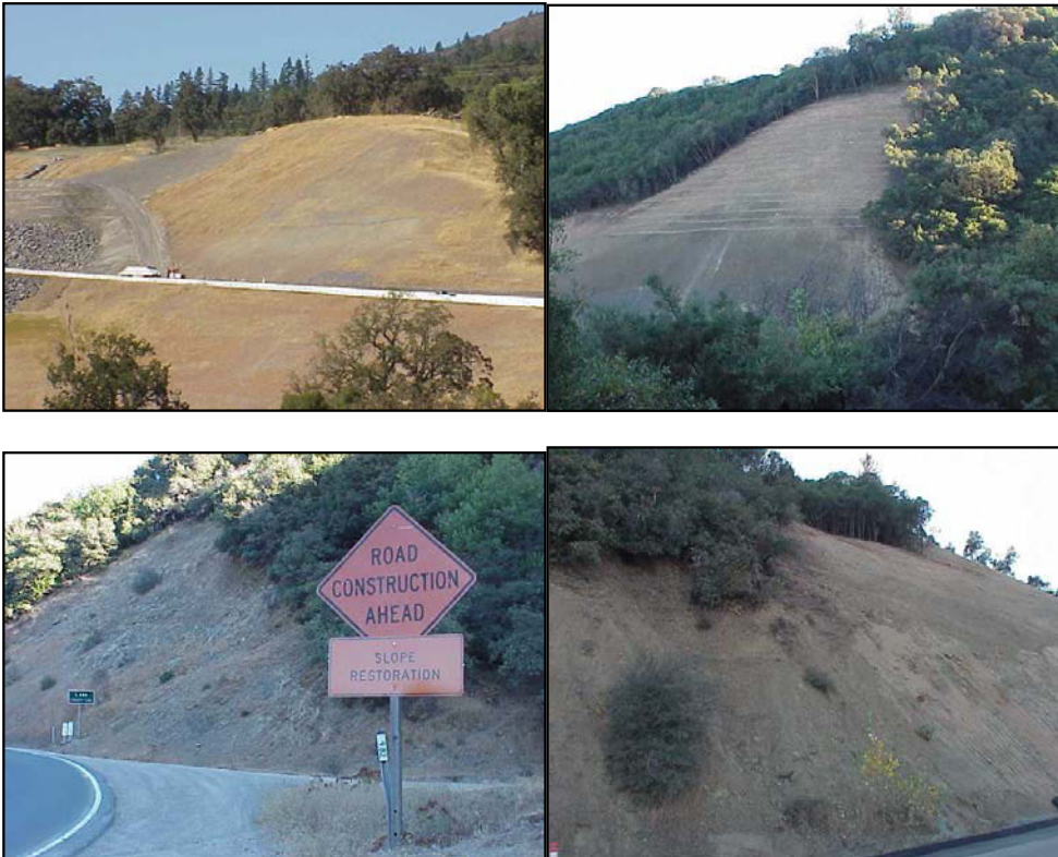
Figure 1. Restoration of severe slopes along highways in Northern California. Photos courtesy of S. L. Young.
