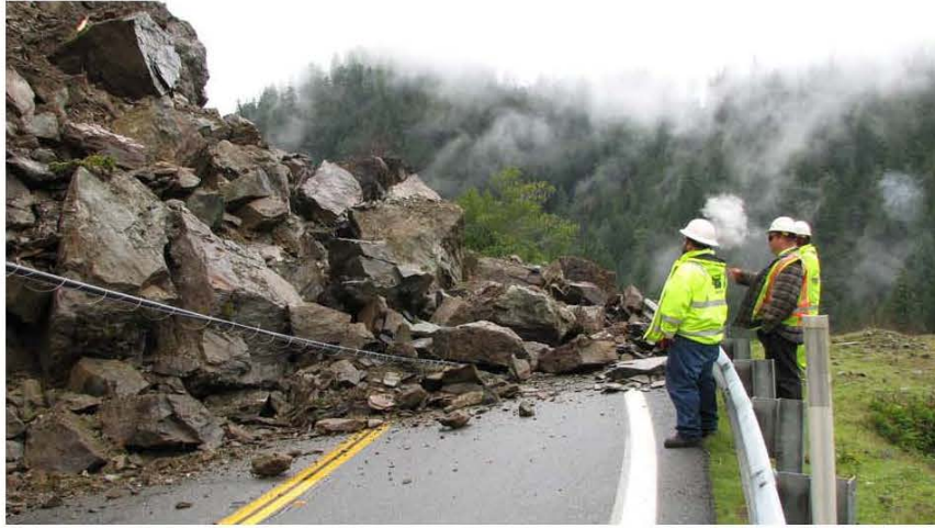
Figure 9: Landslide on SR 96 – Image Courtesy of Caltrans District 1
