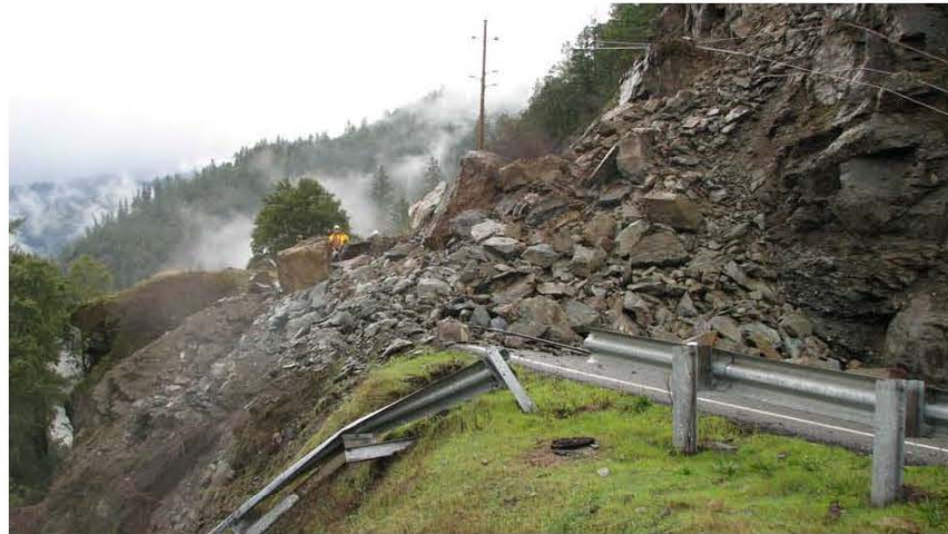
Figure 10: Landslide on SR 96 – Image Courtesy of Caltrans District 1
