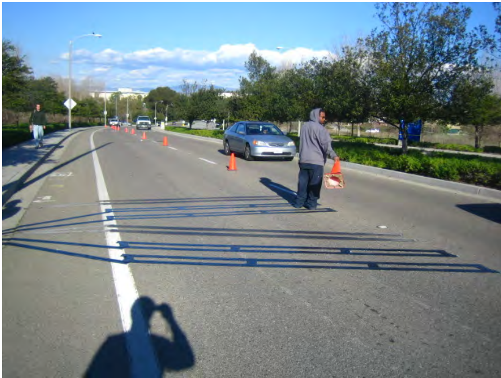
Figure 3-12 Installation of 8-inch Surface Mounted Blade™ Inductive Sensors at Bison Ave Study Site at the University of California, Irvine
