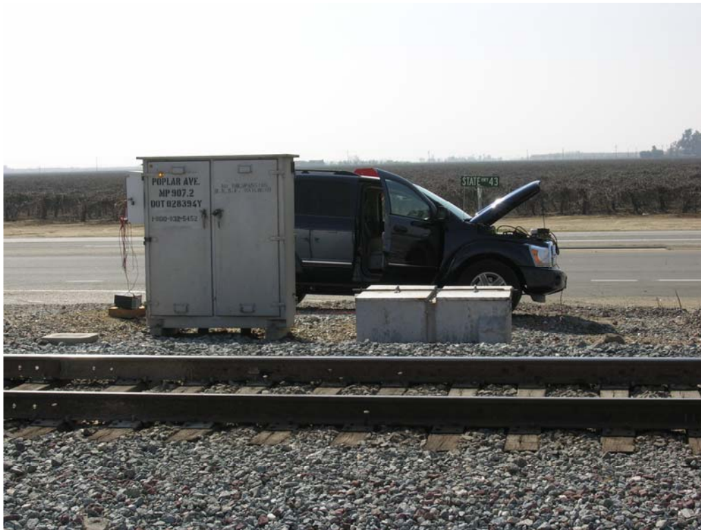
Figure 13: The inverter used to supply AC power is seen resting above the grill on the vehicle. This allowed complete isolation from the AC power in the railroad control box seen on the left.
