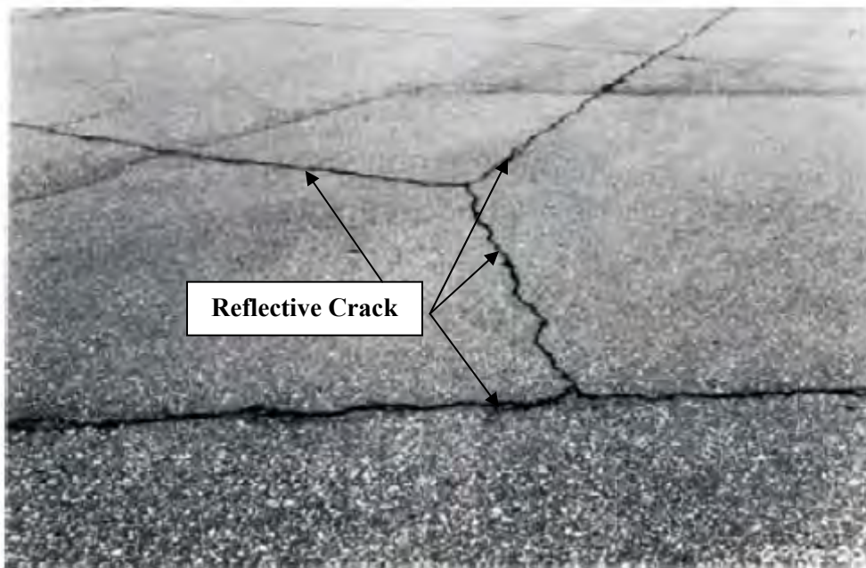
Figure 2-8. Reflective cracking. (Paver - Asphalt Surfaced Airfield)
