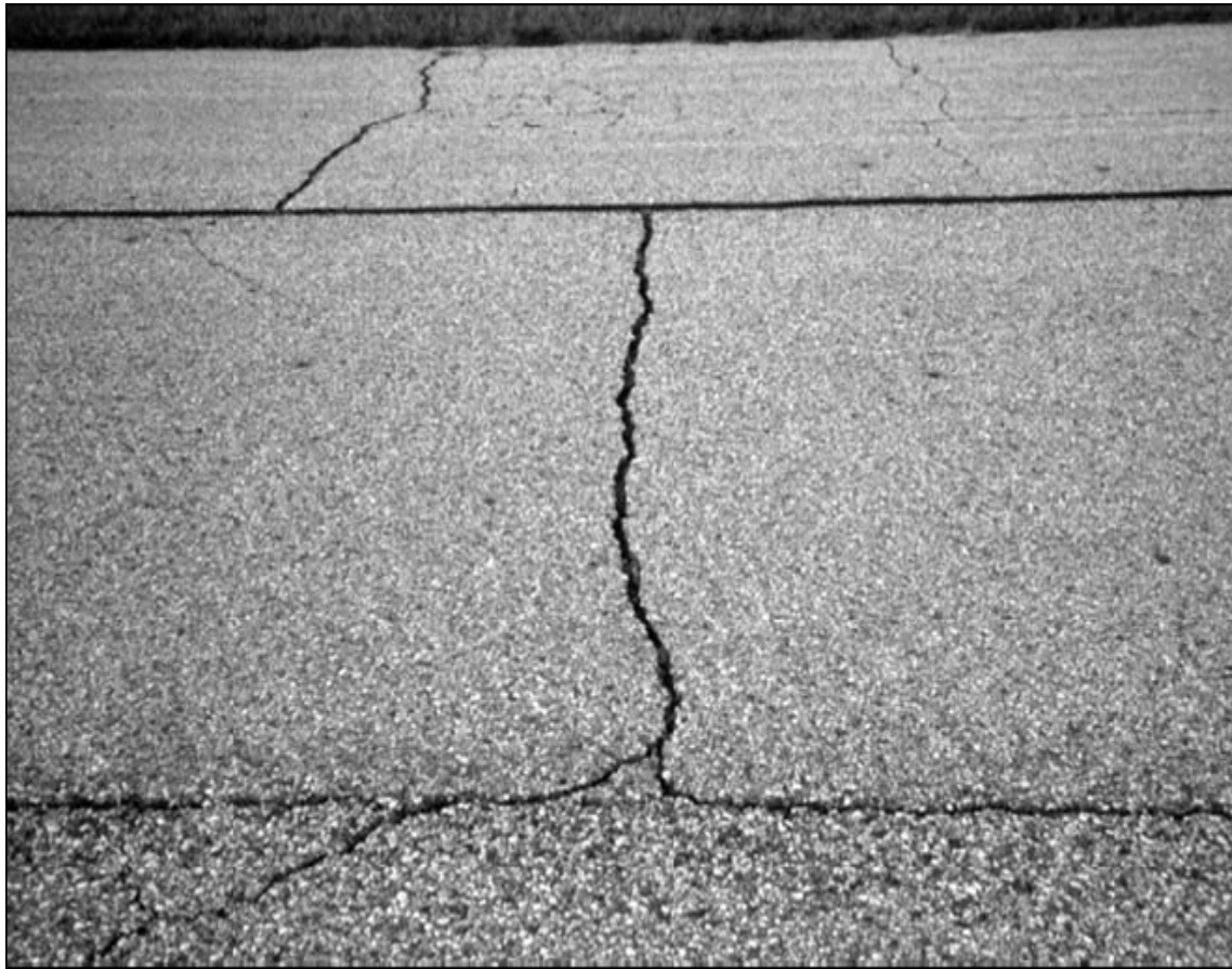
Figure 2-6. Block cracking. ( PASER Manual for Asphalt Airfield Pavements )
