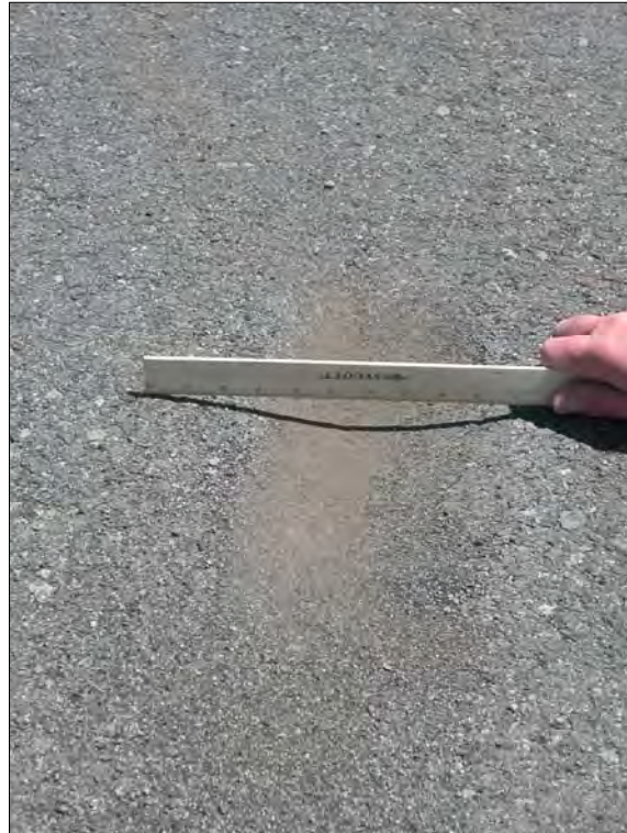
Figure 2-16. Depressed area caused by aircraft parking on HMA before it cooled.
