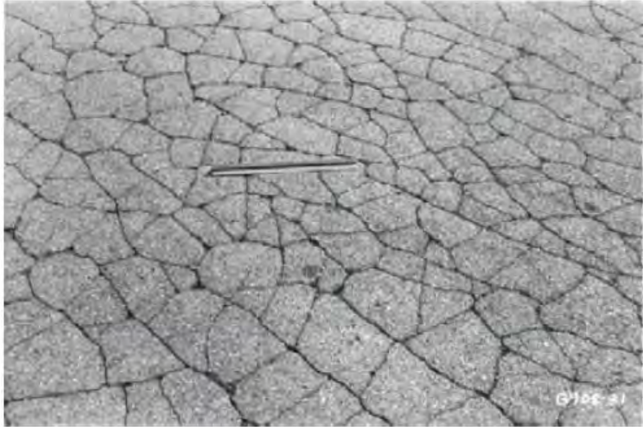
Figure 2-10. Alligator cracking. ( PASER Manual for Asphalt Airfield Pavements )
