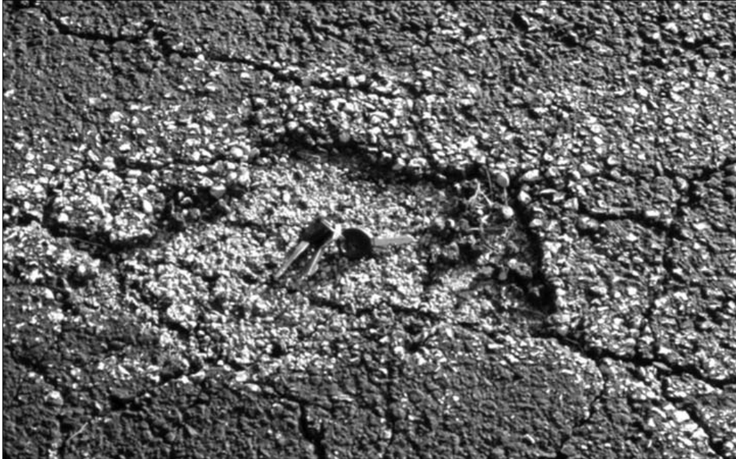
Figure 2-14. Potholes. ( PASER Manual for Asphalt Airfield Pavements )
