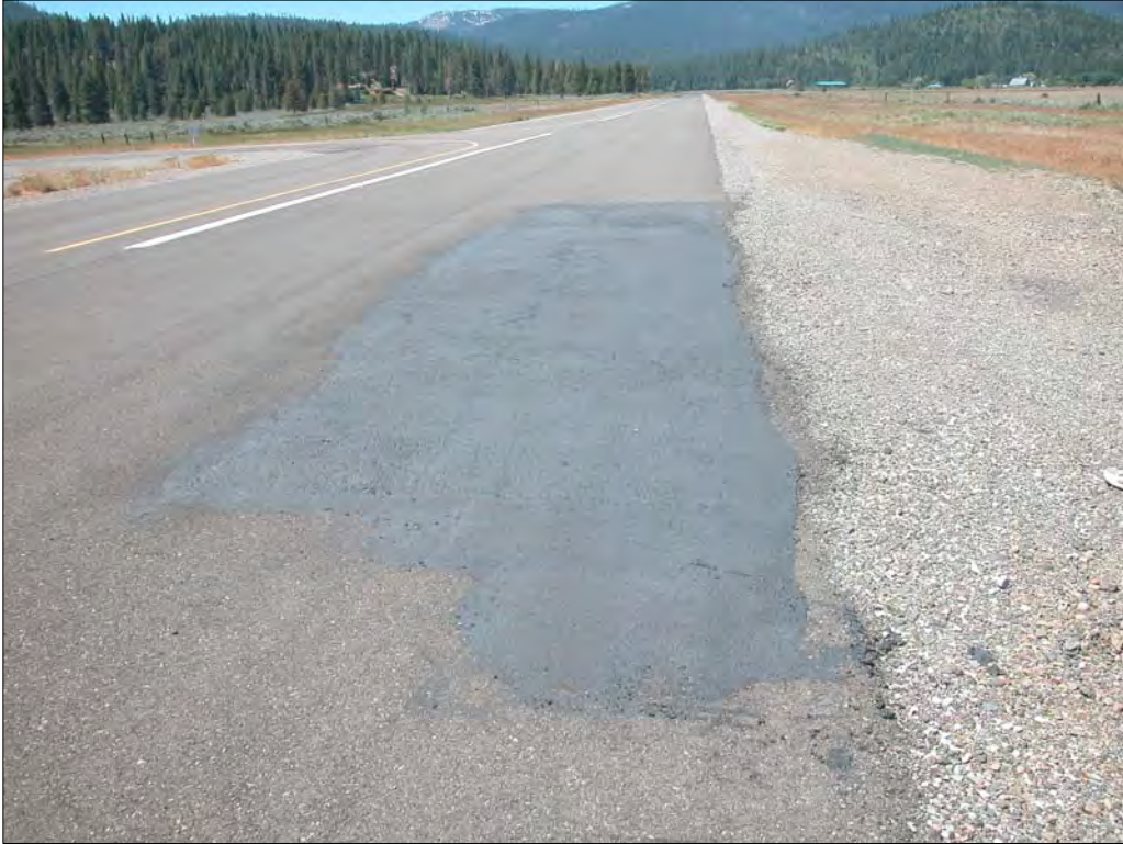
Figure 2-15. Patched depressed area.
