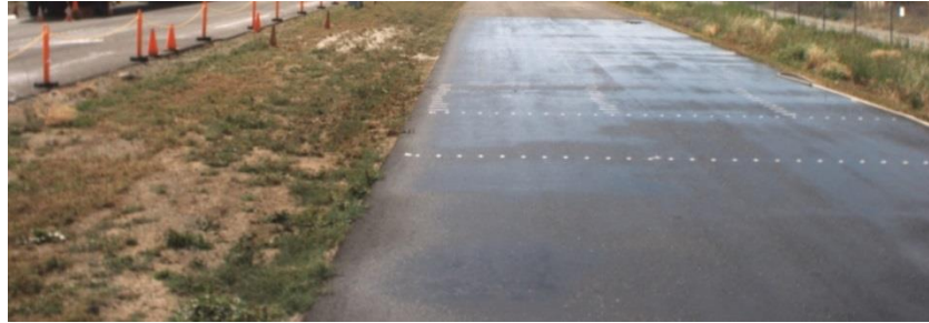
Figure C.1. Front Center Camera view of the wet asphalt pavement
