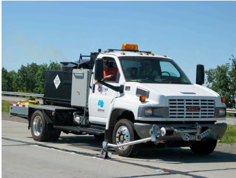
Figure 5. TTLS Appl. Truck Sealing Hwy 113
