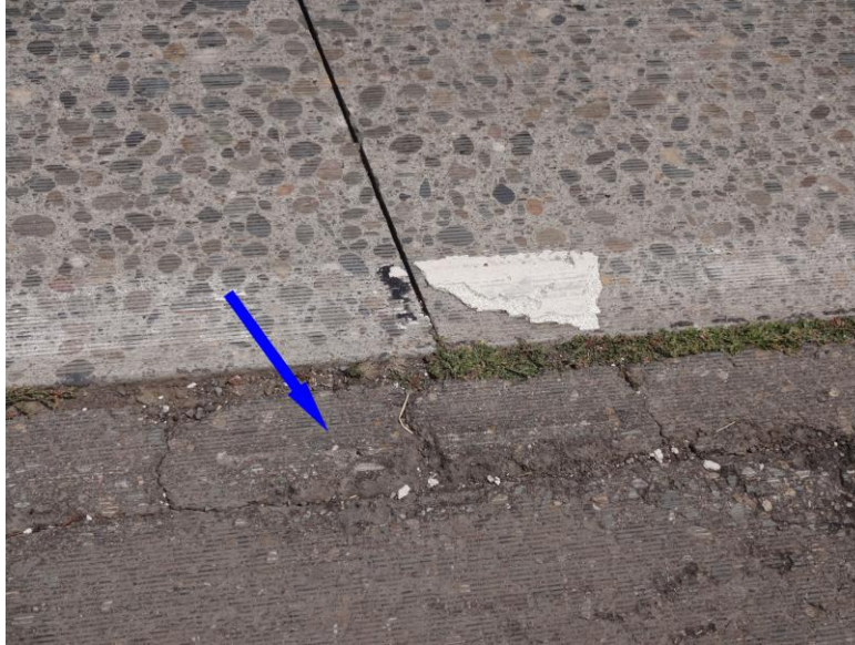
Figure 27. Edge Drain Pavement Failure
