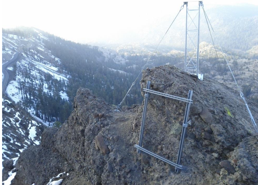
Figure 3.28: The west view of the final site tower installation and electronics enclosure mounting brackets
