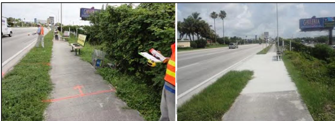
Figure 5. (Left) Bus Stop Before Reconstruction for ADA Accessibility (Right) Bus Stop Following Reconstruction
