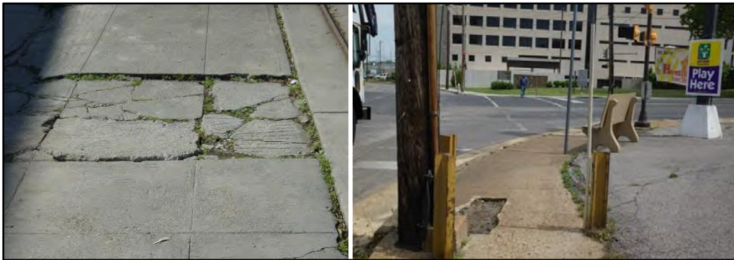
Figure 19. (Left) Uneven, Cracked Sidewalk Surface; (Right) Obstacles Limiting Sidewalk Width and Broken Surface
