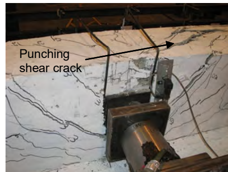
(h) At failure, west bearing detail
