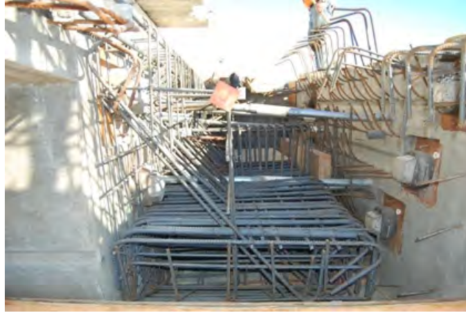
Fig. 2.5 Reinforcement congestion of in-span hinge of prestressed box-girder bridge.
