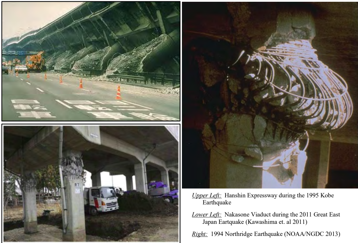
Figure 1-1: Confinement damage to reinforced concrete columns
