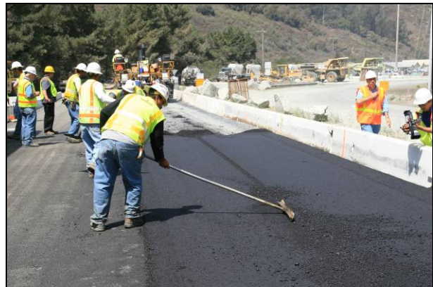
Figure 2.34: Evotherm: Damage repair.
