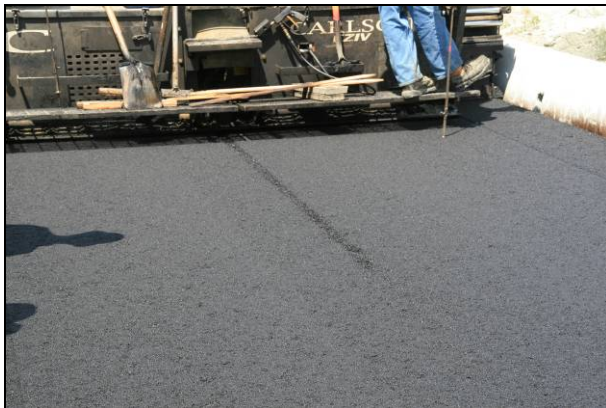
Figure 2.33: Evotherm: Damage behind paver.
