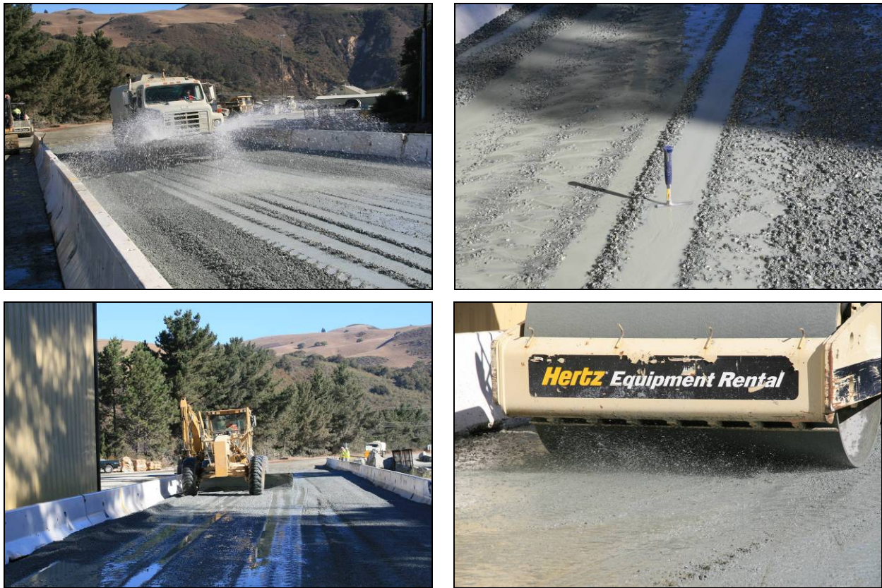
Figure 2.9: Overwatering during base-course construction.
