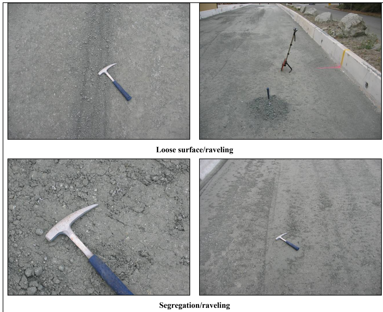
Figure 2.12: Isolated areas of distress on the base-course.
