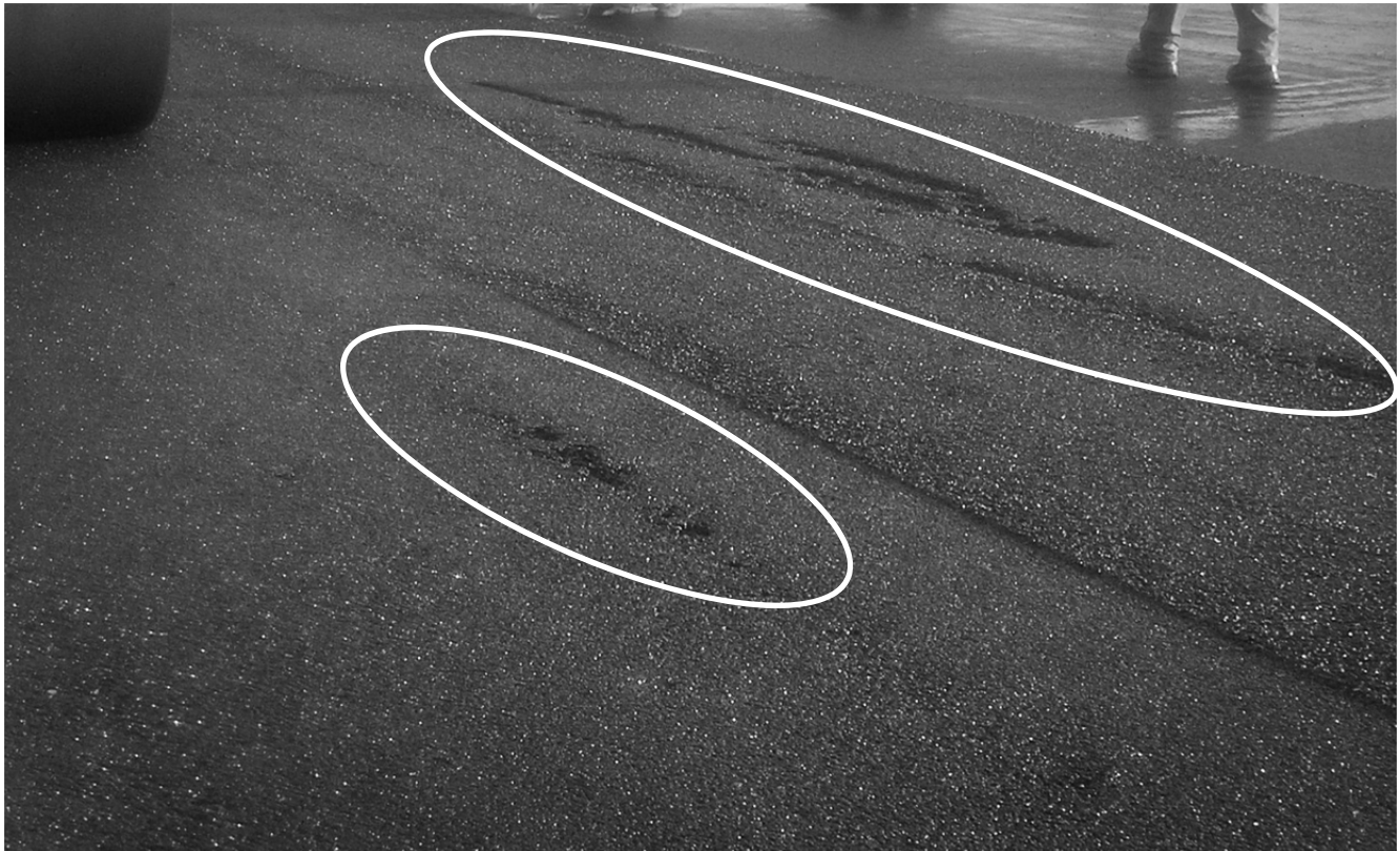
Figure 2.6: Scarring caused by crusted mix (Cell B1, #4P mix with PG 76-22PM).
