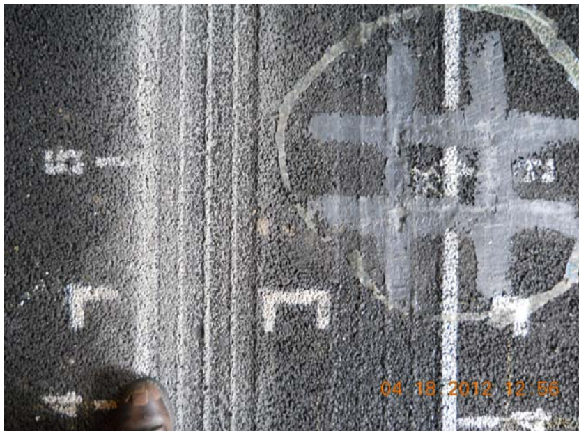
Figure 3.14: Section 653HB after 2,000 load repetitions with the asphalt concrete block at Station 5.
