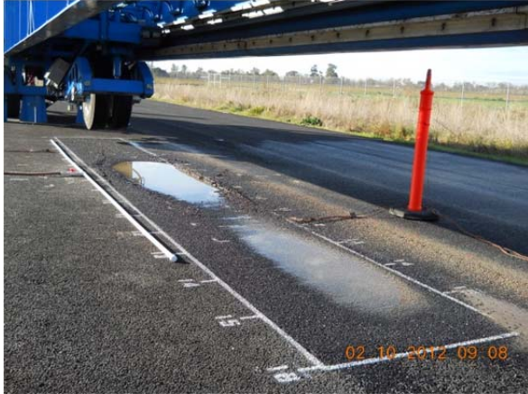
(a) Overall view of the failed pavement
