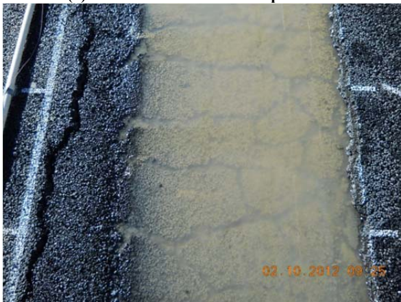
(c) Severe cracking and punch down near Station 7
