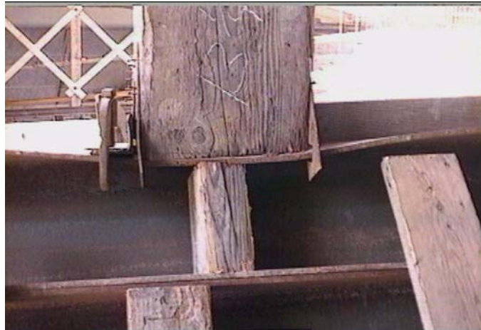
FIGURE 1-3 Localized flange bending failure in sill beam (J. Lammers, Caltrans, Personal communication)
