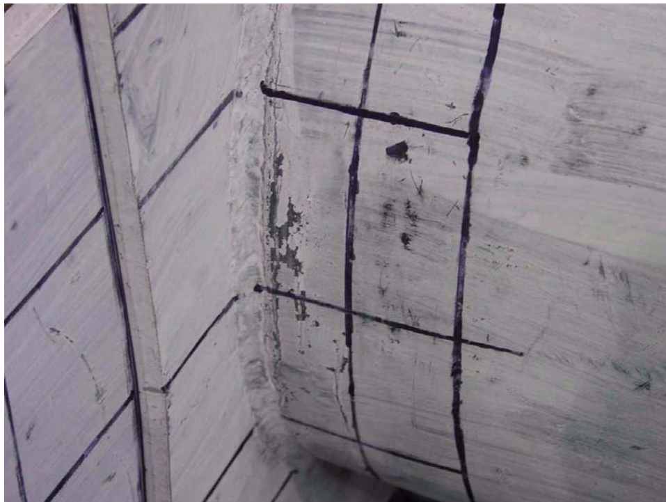
FIGURE 2-37 Onset of yielding and buckling in the steel post for 1490SPNBTCRE0 - Beam 2
