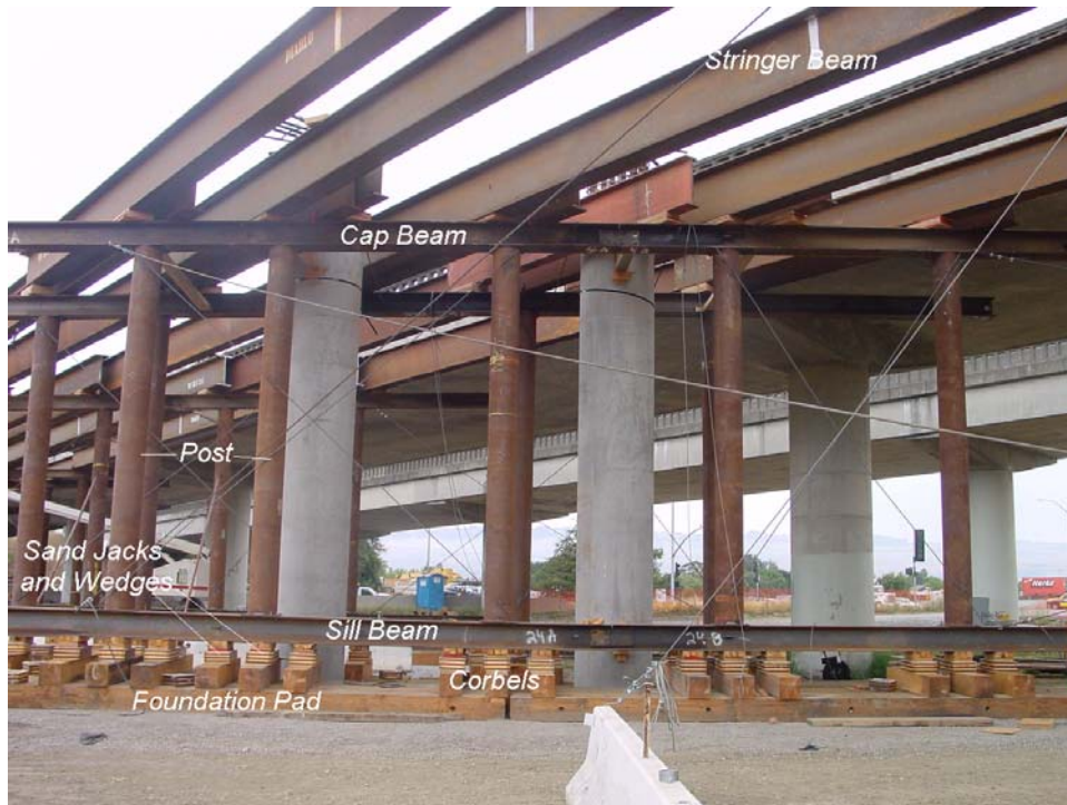
FIGURE 1-1 Bridge Falsework for the Petaluma River Bridge at the intersection of California State Routes 101 and 116
