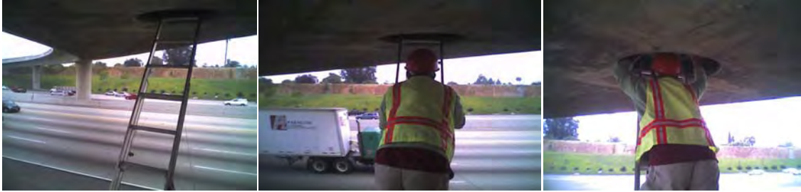
Figure 3. Access to the monitoring system inside the box girder at WSO Bridge.
