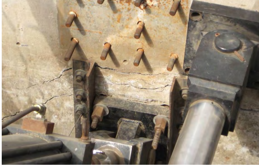
Figure 3.7 Abutment Wall Cracks Between Actuators 2 and 3L
