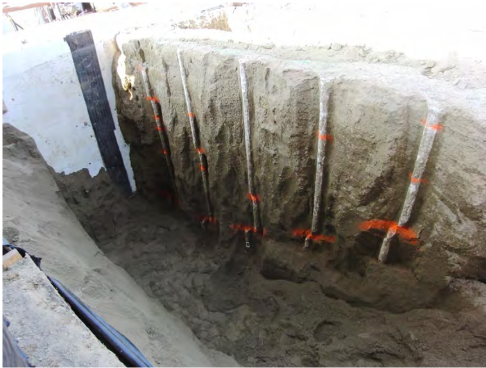
Figure 5. 40 Photograph showing the initiation of the major failure surface at the bottom of the wall for T8.0-1
