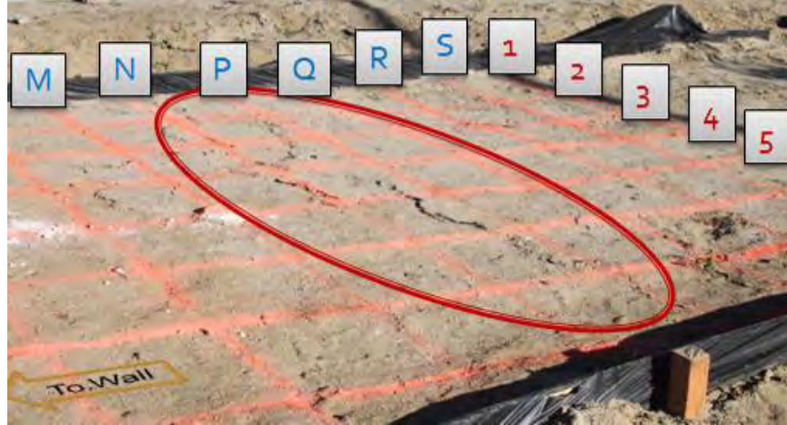
Figure 5. 36 Main Failure Surface Crack after T8.02c
