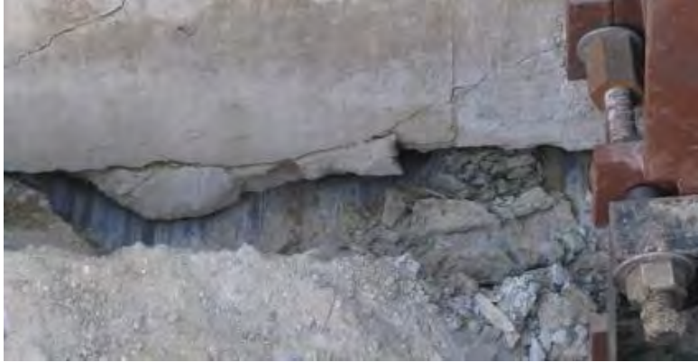
Figure 5. 11 Visible striations on the steel base plate during T8.0-2b and T8.0-2c indicating movement along the wall-grout-plate interface
