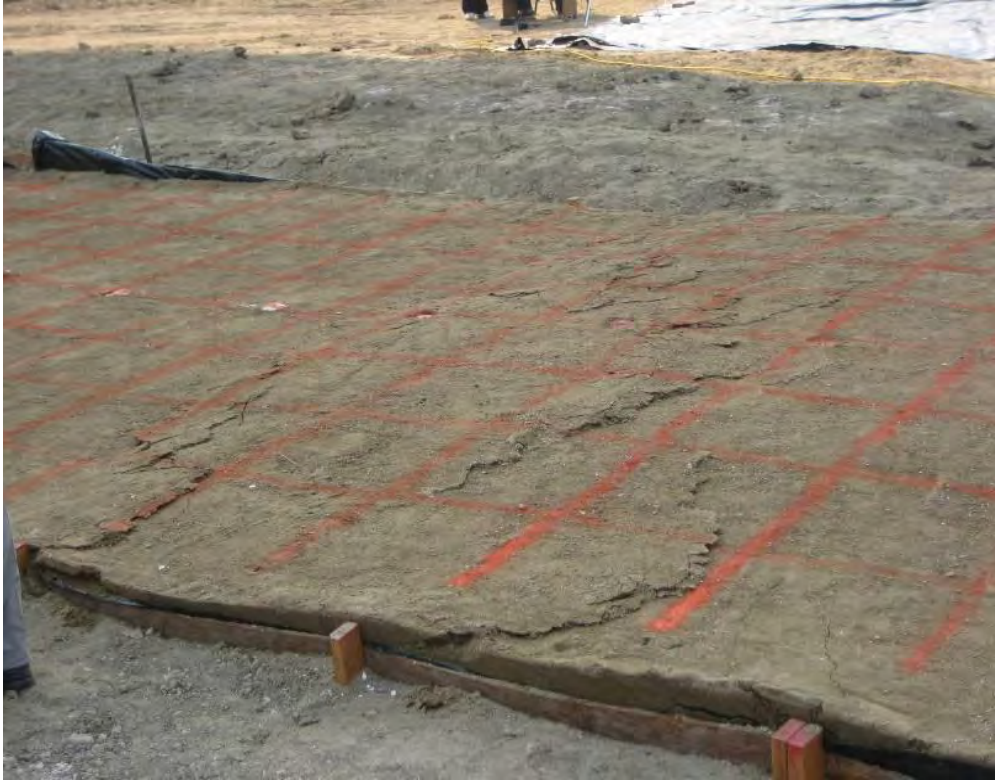
Figure 5. 31 Backfill upheave and major cracking at the location where the principal failure plane intersects with the surface
