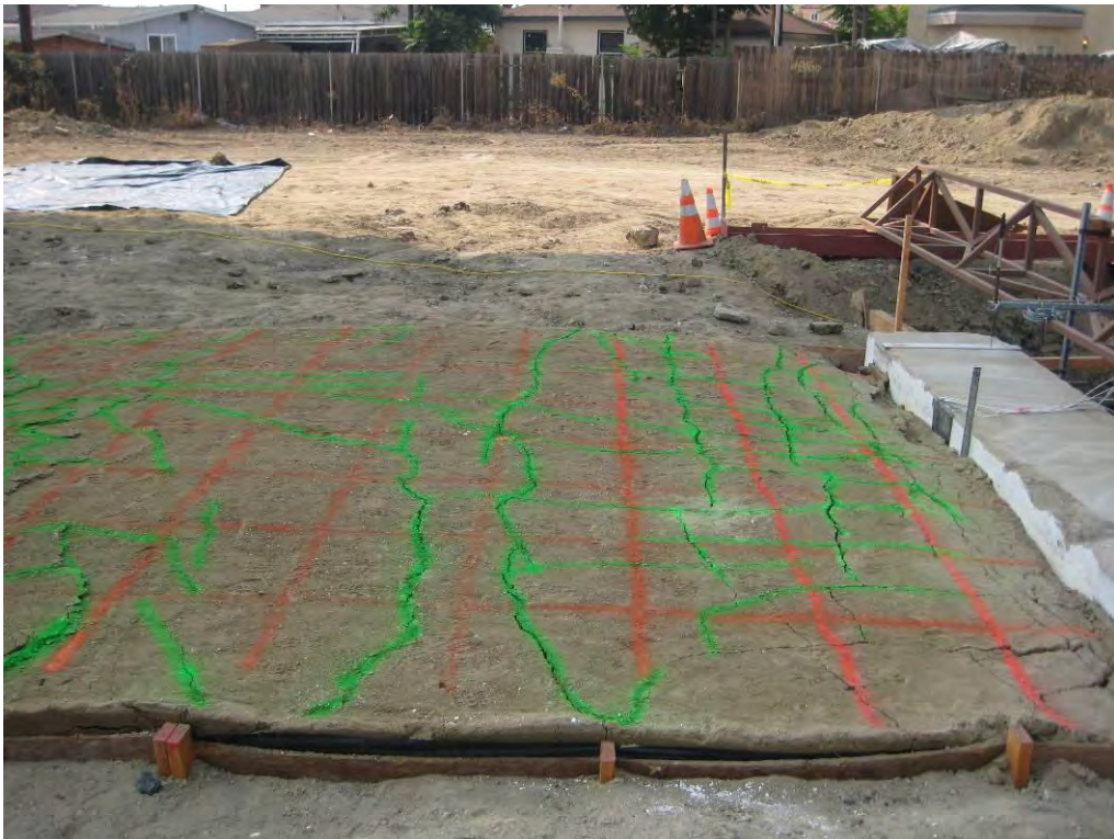
Figure 5. 30 Surface cracks on the backfill of T8.0-1 marked in green color
