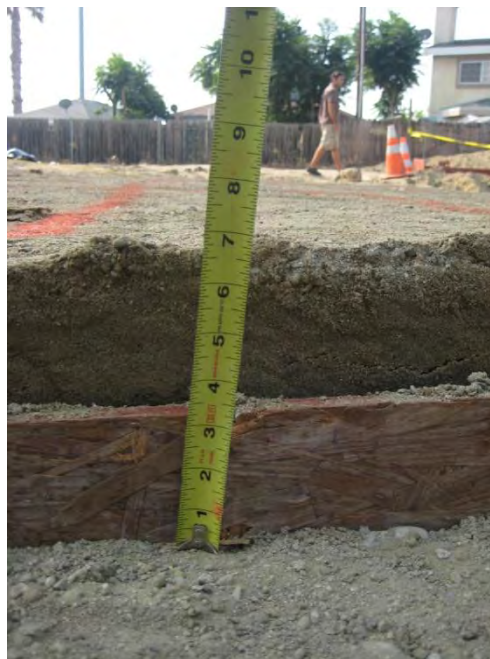
Figure 5. 32 Photograph of backfill upheave along the wingwalls of the specimen
