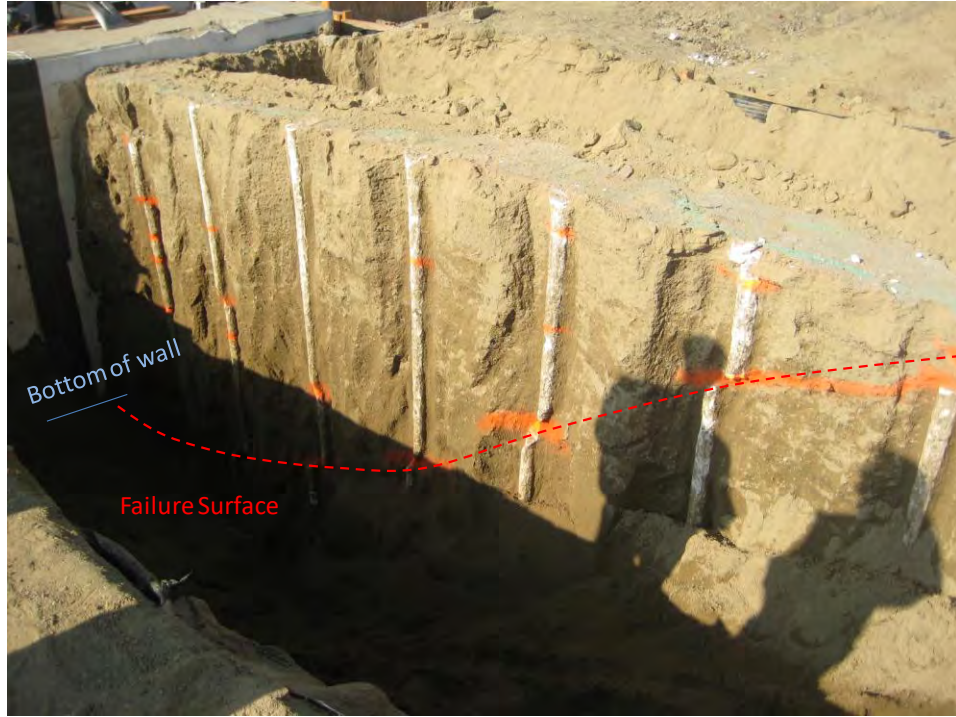
Figure 5. 39 Trace off failure surface observed for T8.0-1
