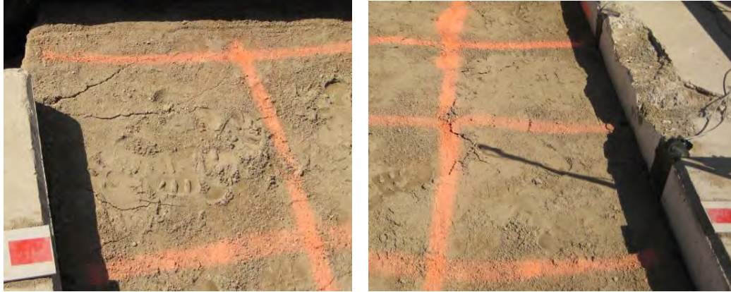
Figure 5. 34 Surface Cracks after test T8.0-2a. Left: Cracking near Grid A-1, Right: Cracking near Grid B-3
